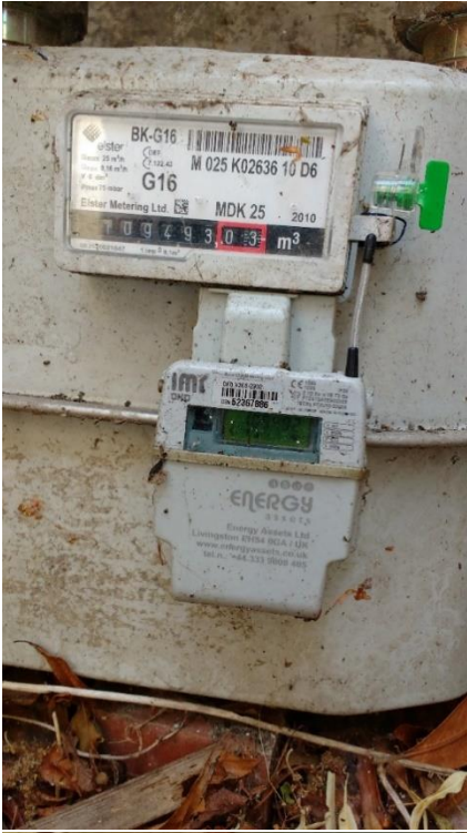
The gas meter is fitted with a smart meter interface.
