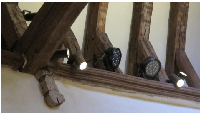
Figure 6 Two types of lighting installed in the nave
