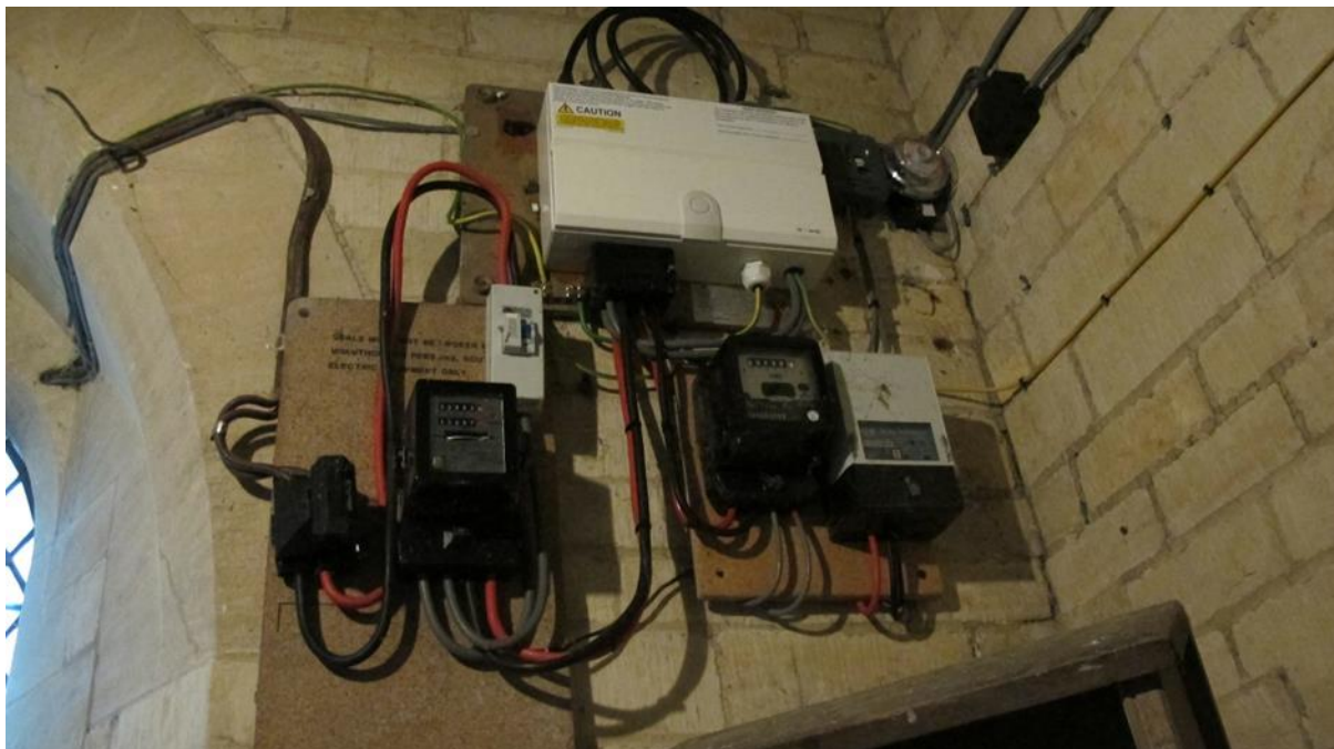
Figure 1 Electricity meters for church and floodlighting.
