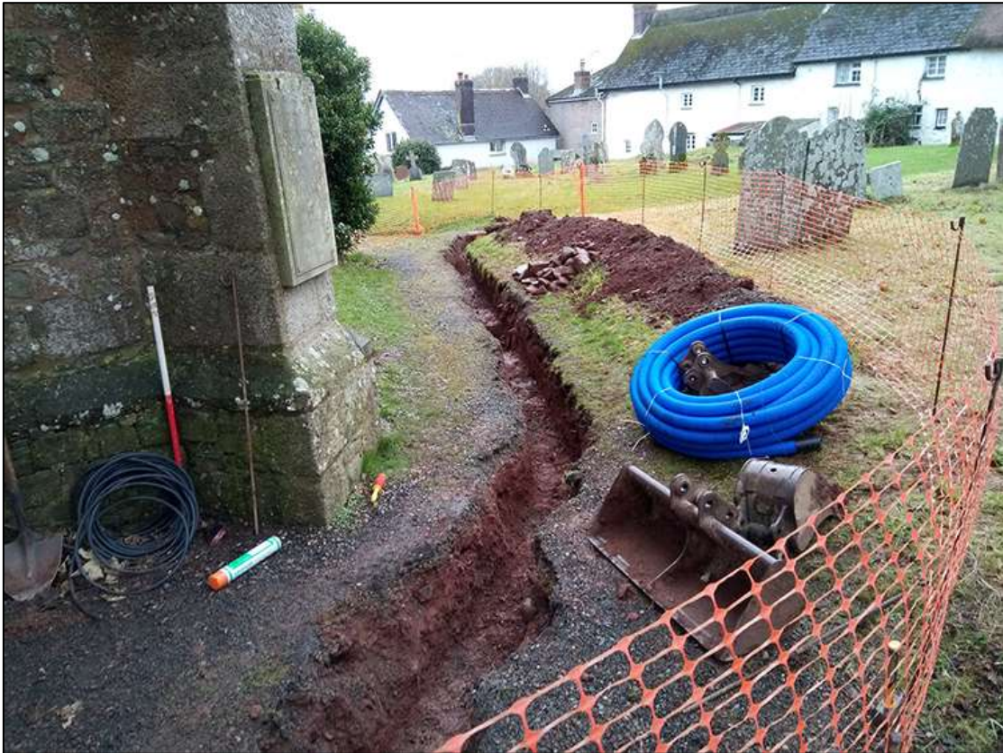
13. EXCAVATED TRENCH SOUTH OF NAVE AND TOWER, POST-EXCAVATION; VIEWED FROM THE NORTH-WEST (1M SCALE).
