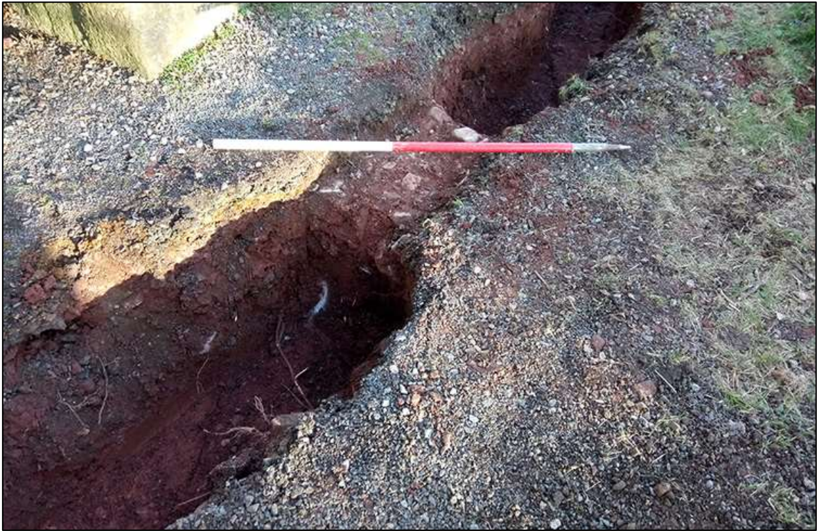
FIGURE 5: CONSTRUCTION CUT [113] AND FOUNDATION WALL {114}, MID-EXCAVATION; VIEWED FROM THE WEST (1M SCALE).
