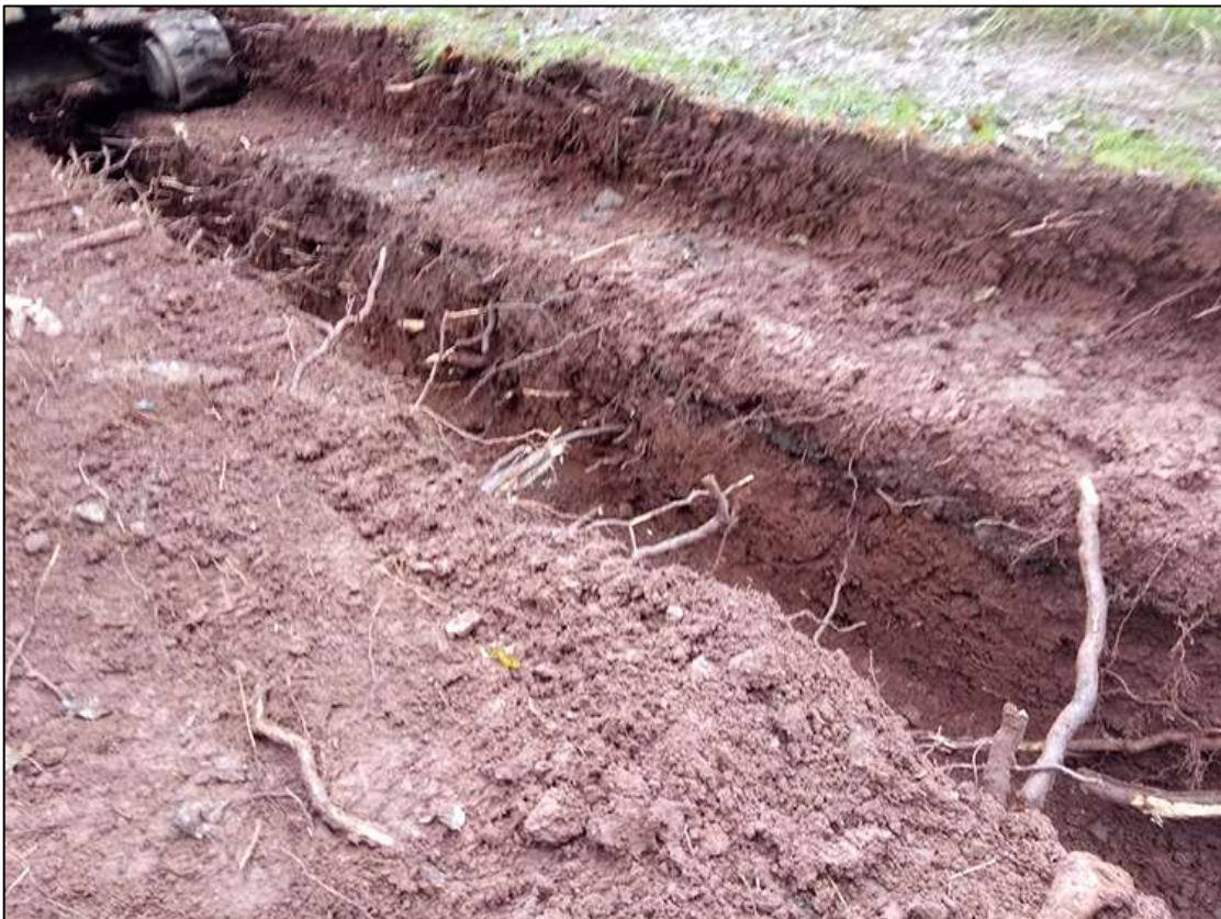
18. AREA WEST OF TOWER, IN RAMPED PATH LOCATION, SHOWING LAYER (104) AND (105) AND ROOT DISTURBANCE; VIEWED FROM THE NORTH-WEST (NO SCALE).
