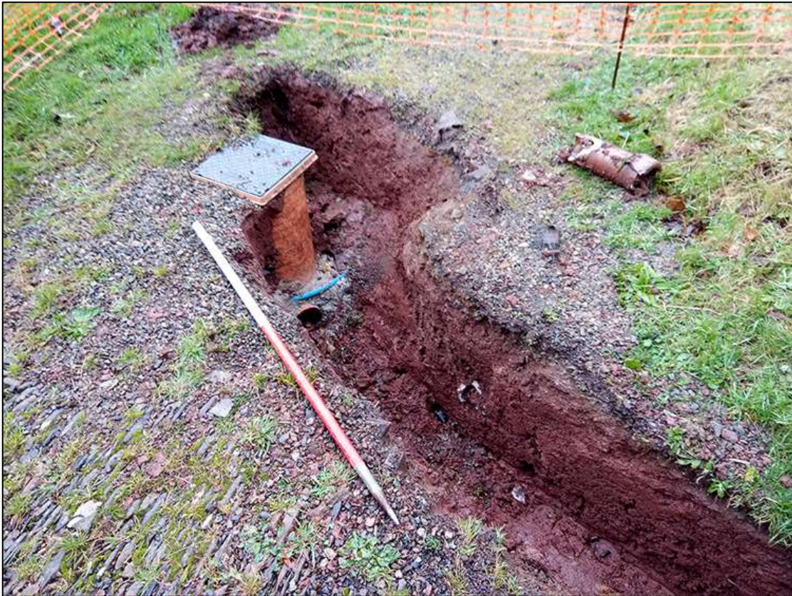
1. EAST END OF EXCAVATED TRENCH, SOUTH OF PORCH, SHOWING MODERN SOAK-AWAY ACCESS; VIEWED FROM THE NORTH-WEST (1M SCALE).
