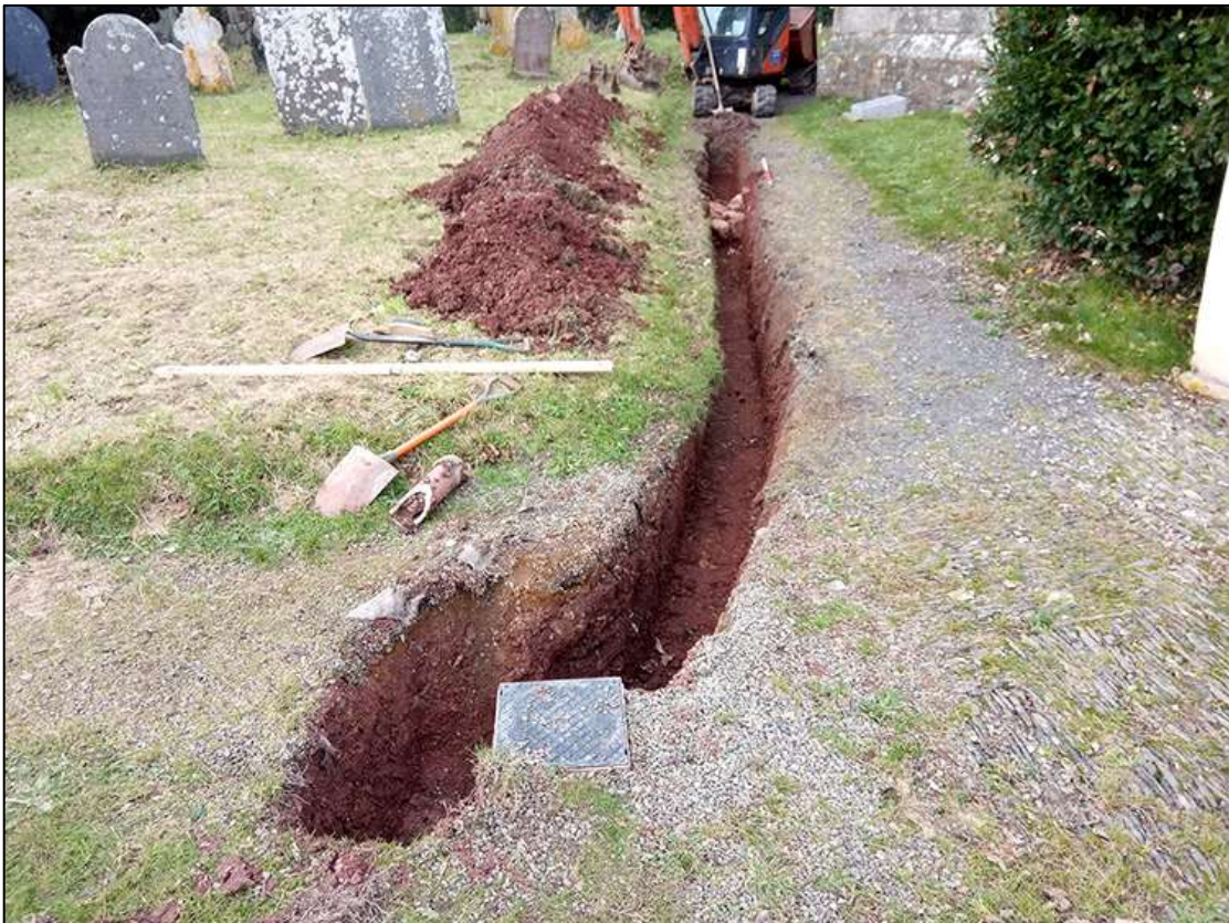
2. EXCAVATED SERVICE TRENCH, MID-EXCAVATION, SHOWING {110} IN DISTANCE; VIEWED FROM THE EAST (1M SCALE).
