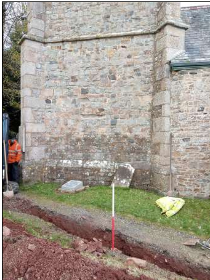
8. APPROXIMATE LINE OF WALL FOUNDATION {110}, TOWARDS TOWER; VIEWED FROM THE SOUTH-SOUTH-EAST (1M SCALE).
