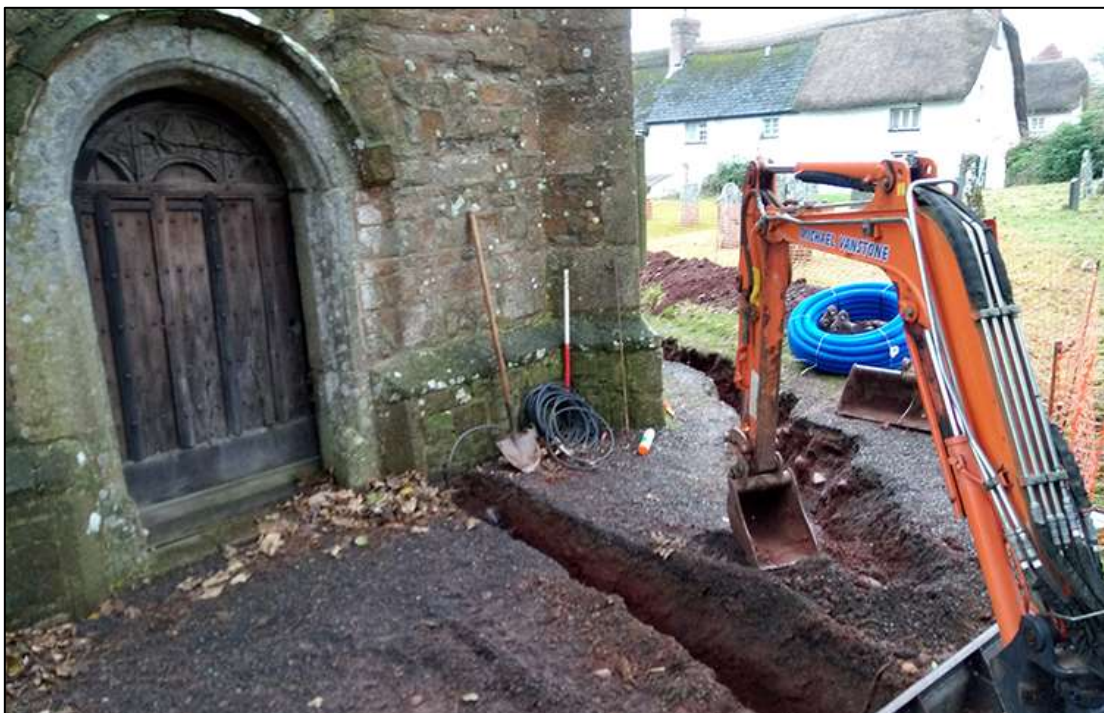
FIGURE 2: AREA WEST OF TOWER, SHOWING LAYERS (105) AND (106); VIEWED FROM THE NORTH-WEST (1M SCALE).
