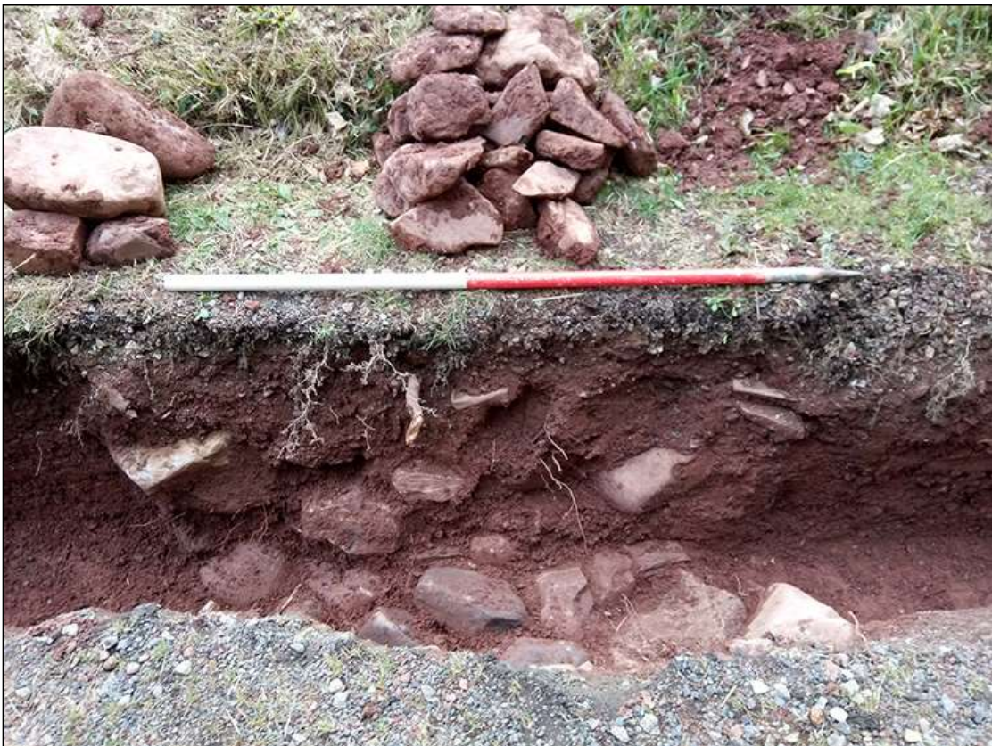
6. WALL FOUNDATION {110}, MID-EXCAVATION TO FORMATION LEVEL; VIEWED FROM THE NORTH (1M SCALE).
