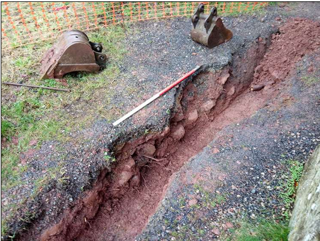
12. SECTION OF WALL FOUNDATION {114} FURTHER FROM TOWER, POST-EXCAVATION; VIEWED FROM THE EAST (1M SCALE).
