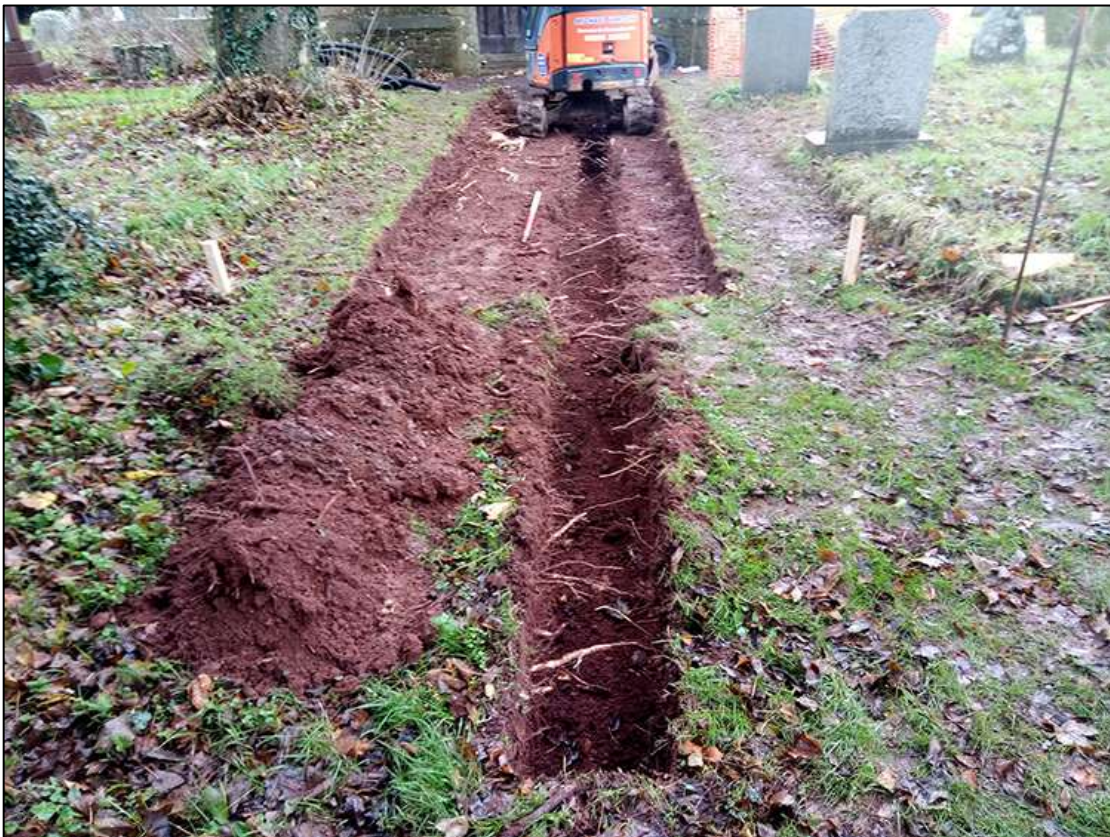
16. EXCAVATED AREA AND TRENCH WEST OF TOWER; VIEWED FROM THE WEST (1M SCALE).
