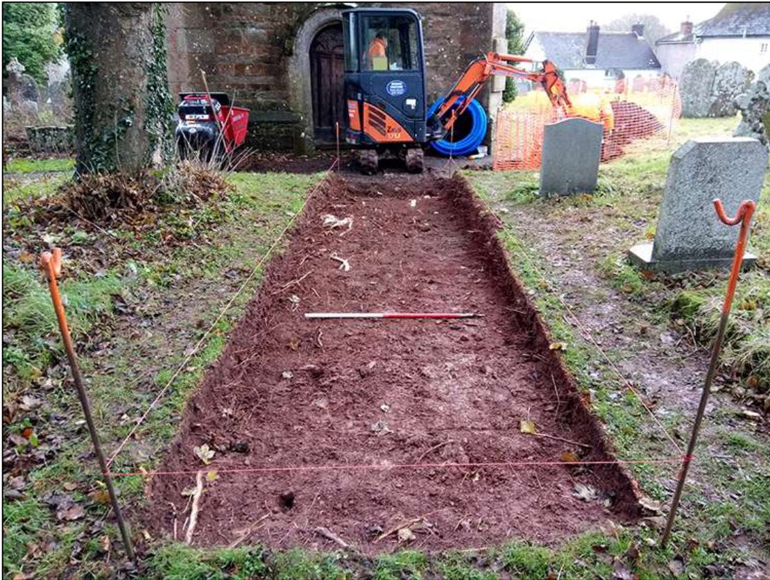
15. EXCAVATED AREA FOR PROPOSED RAMPED FOOTPATH; VIEWED FROM THE WEST (1M SCALE).
