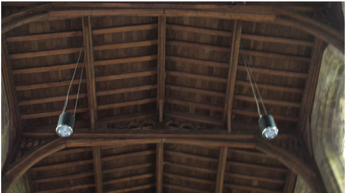
Figure 3 Mercury vapour lamps at front of nave. Note the low pitch roof
