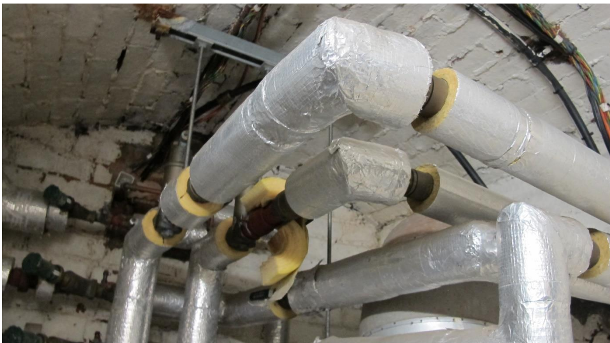
Figure 12 Sections of pipe and valves are not lagged
