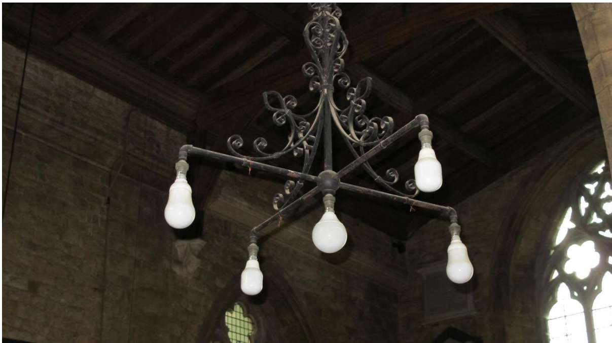
Figure 1 Nave lighting is provided by 8 sets of 5 bulbs
