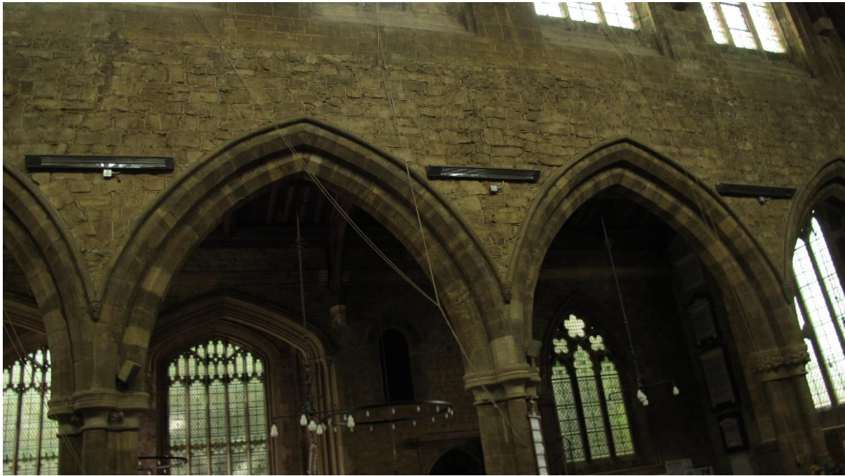
Figure 13 Location of existing radiant heaters in nave
