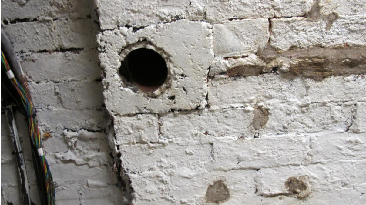
Figure 10 Presumably an old flue hole, above the boiler, probable source of the water.
