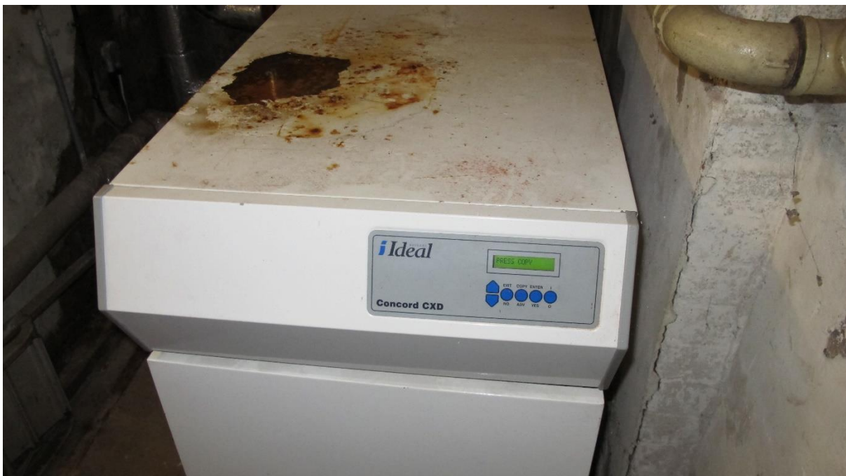
Figure 9 Existing boiler; the Ideal Concord range is listed as having an efficiency of 76%.
