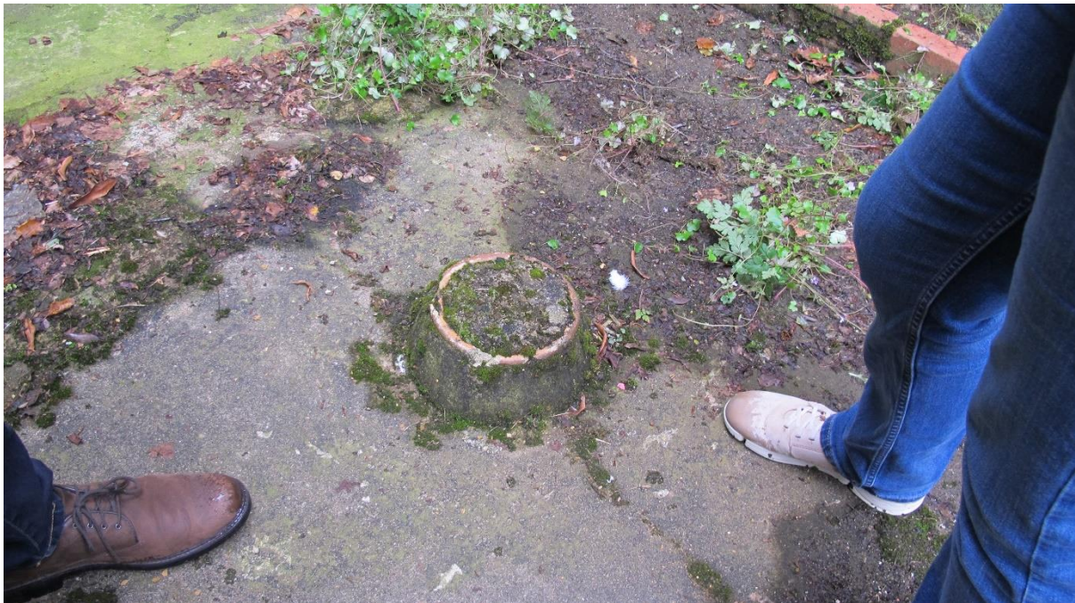
Figure 11 External evidence of former flue
