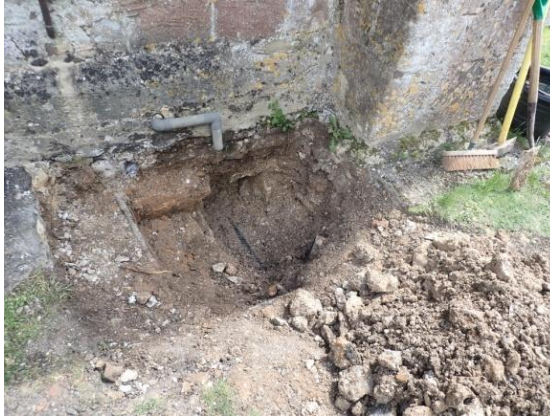
Plate 30: Hand excavations at the west wall of the west tower, from the west
