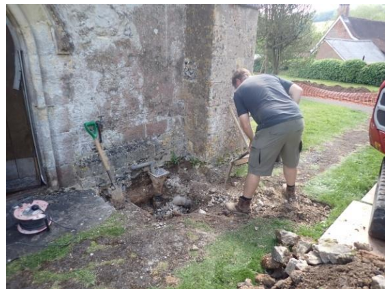
Plate 28: Hand excavations at the west wall of the west tower, from the north
