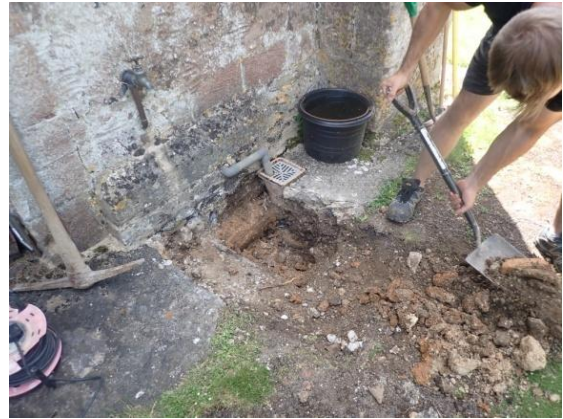
Plate 27: Hand excavations at the west wall of the west tower, from the north
