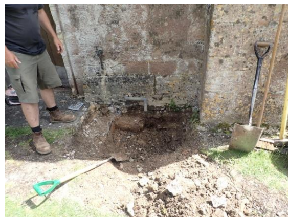
Plate 29: Hand excavations at the west wall of the west tower, from the west
