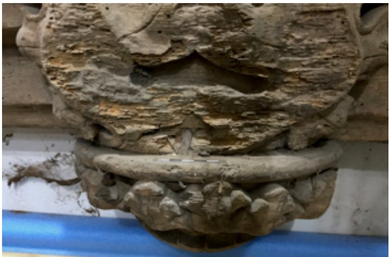
Figure 15 ~ Decay and surface loss to Beam corbel on Truss 1. Note iron fixing securing the base of the corbel to the beam.
