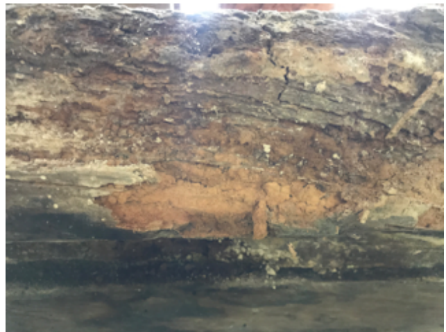
Figure 13 ~ Area of decay caused by prolonged damp. Attempts at past repair are evident, however the damp was on-going. The orange indicates more recent surface loss.
