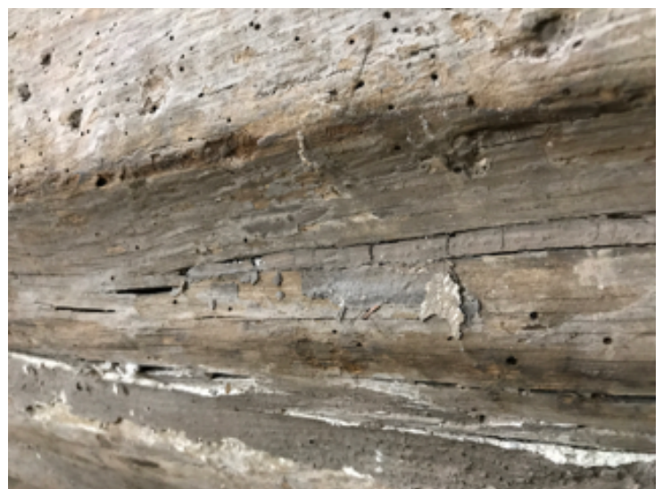
Figure 37 ~ Brown paint over truss and plaster repair within the shakes of the truss.
