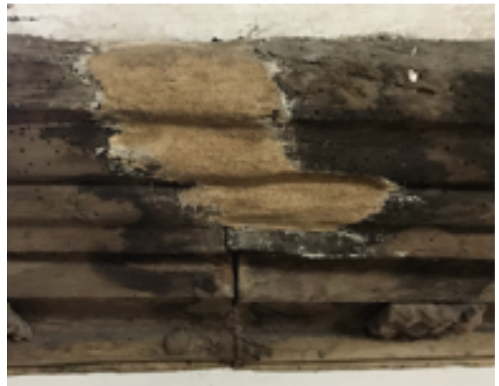
Figure 21 ~ Boss FBN1 with soft plaster fill applied to void between boss and purlin. The fill is cracked and loose.
