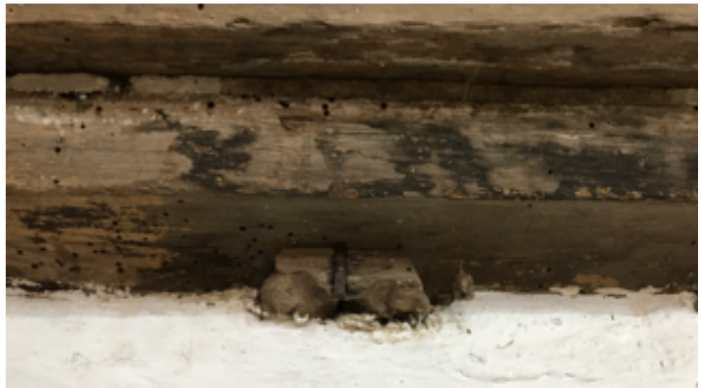
Figure 33 ~ Detail of Bay 3 north elevation and paterae P3N1 which is half missing.
