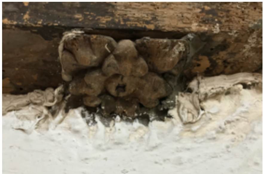
Figure 25 ~ Detail of patera P3N2 which is partially concealed by poorly applied repair.
