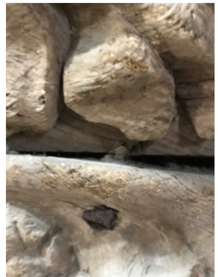
Figure 28 ~ Iron fixing through base of beam corbel 5 into tie beam.
