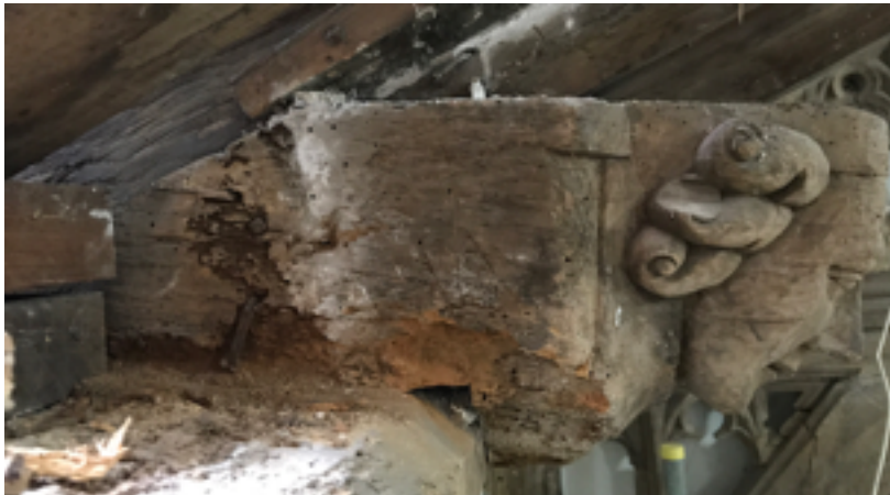
Figure 26 ~ Corbel CN5 illustrating timber decay and loss to rear. Note corroding iron fixing into wallplate.
