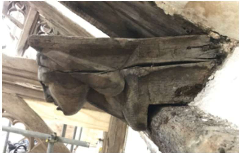
Figure 18 ~ Corbel CS1 illustrating historic shake extending from the rear to the front face. The corbel has suffered from damp and is disfigured with dark water stains but is not deemed unstable
