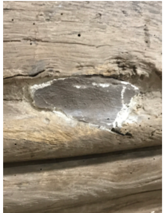
Figure 11 ~ Plaster repair painted the same brown as seen over the Truss painted area.
