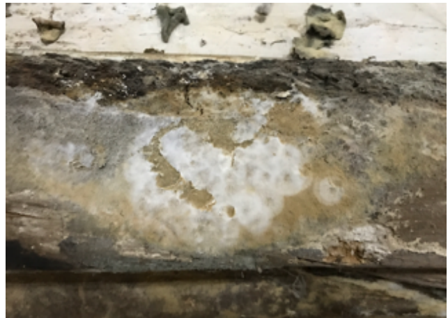
Figure 12 ~ Area of mould over a lime plaster fill on the wallplate. Note the brown paint to the right over the plaster.
