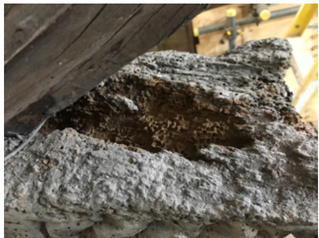
Figure 14 ~ View from above of a corbel illustrating the insect damage of the internal timber.
