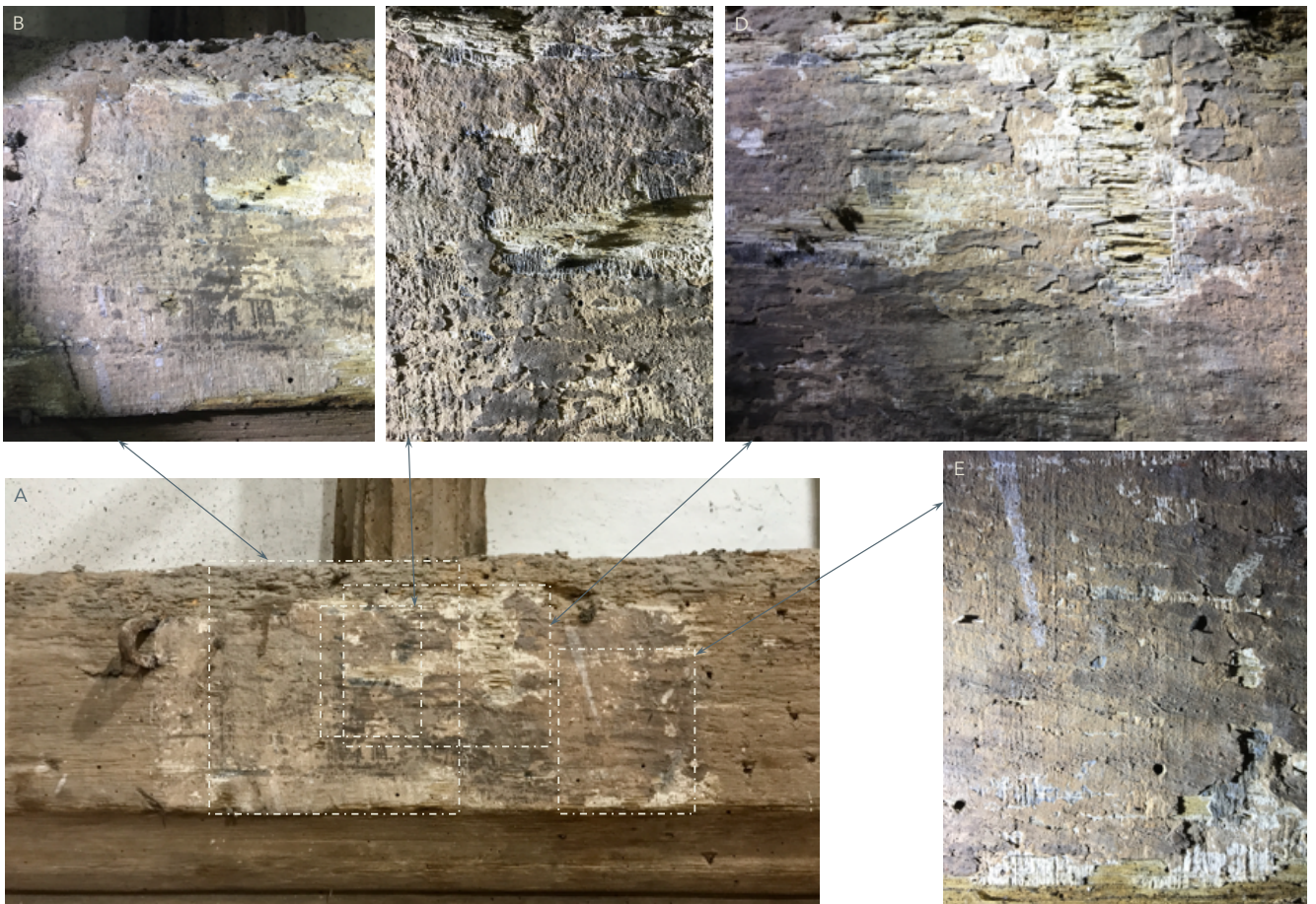
Figure 9 ~ Painted patch on Truss 6. Image A shows the area of the applied paint. Images B, C, D and E were taken in raking light to illustrate the application of the paint and highlight the different layers.
