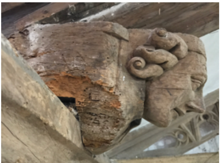
Figure 17 ~ Recent loss of decayed area to corbel CN5 (exposed orange).
