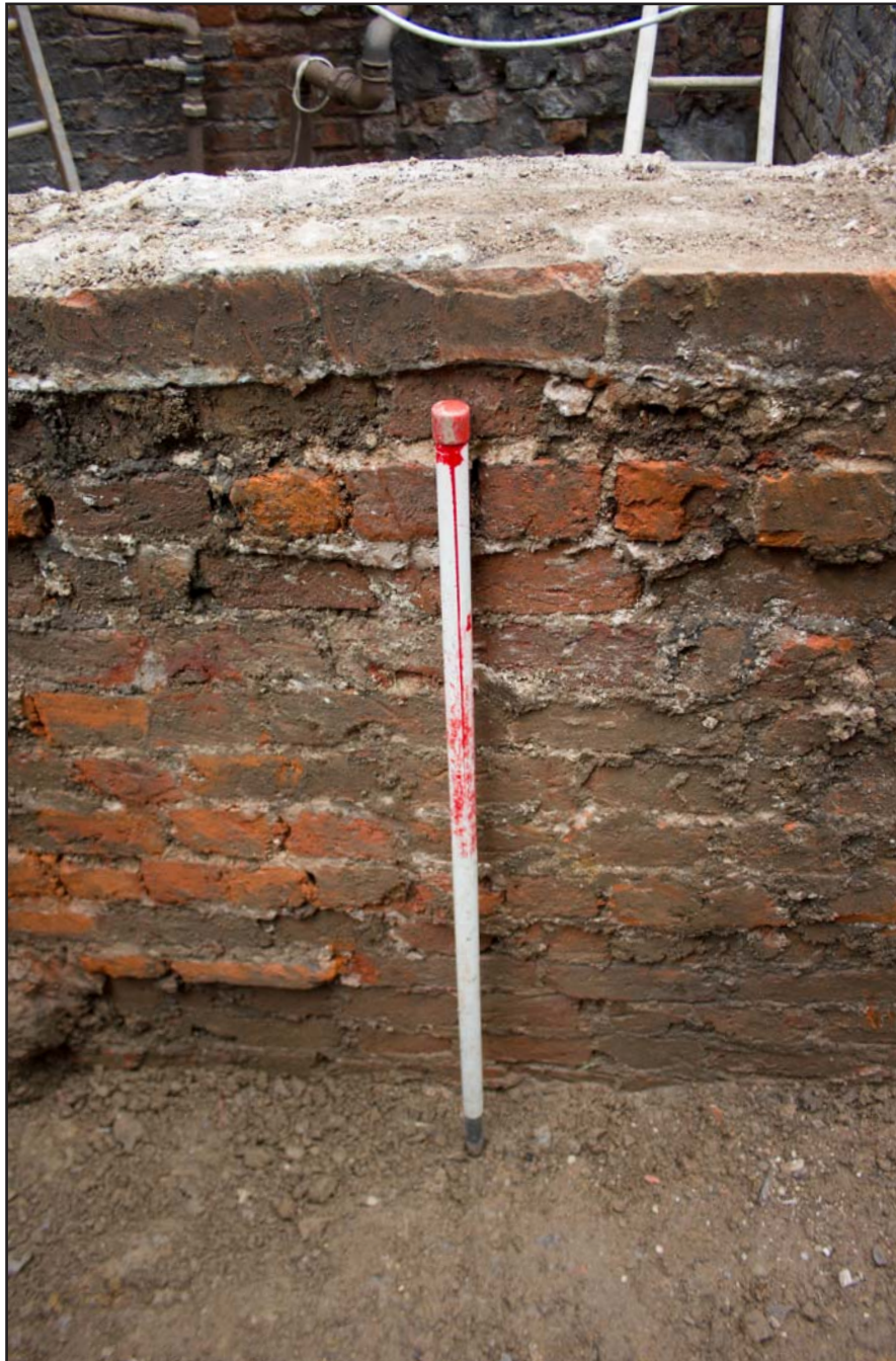
Plate 13: Section of Trench 3 showing elevation of previous boiler room red brick wall at St. Mary's Church, Bosley, Macclesfield - from the west - scale 1m
