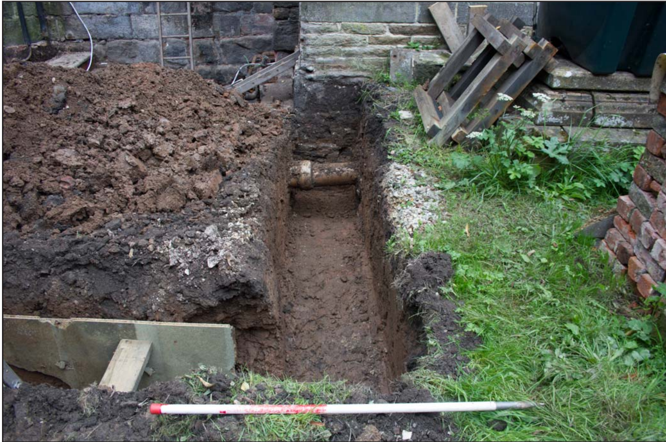
Plate 03: Trench 1 post excavation at St. Mary's Church, Bosley, Macclesfield - from the south - scale 1m
