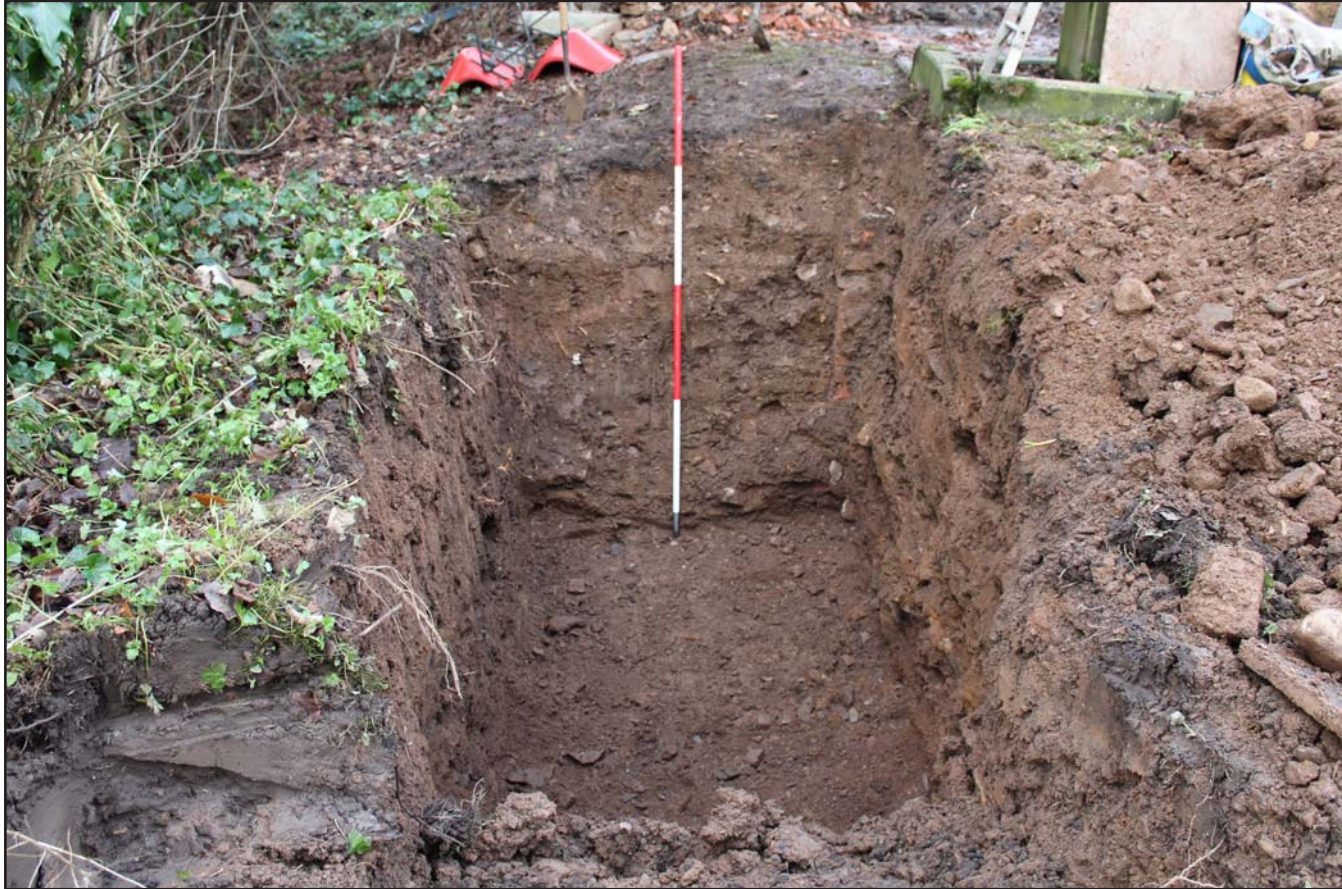
Plate 17: Post excavation of area for sump at St. Mary's Church, Bosley, Macclesfield - from the south - 2m scale
