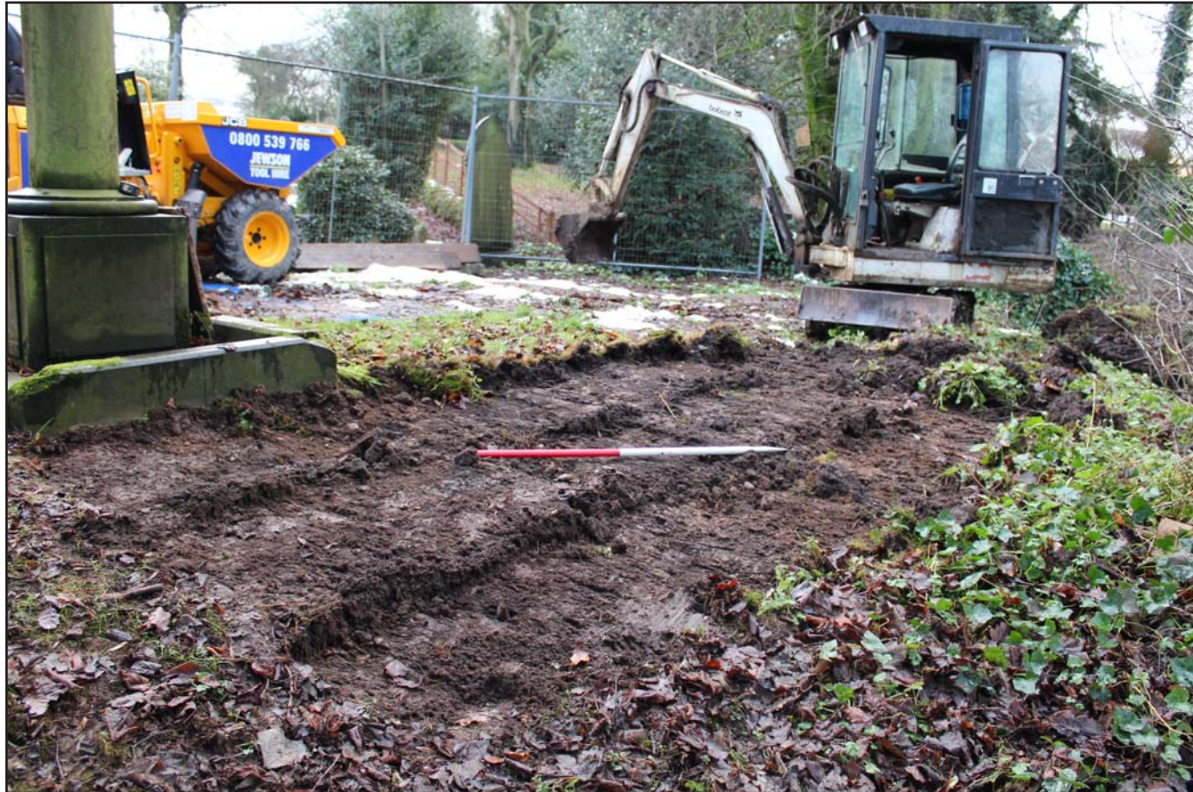
Plate 15: Pre excavation shot of area for sump and drainage trenches at St. Mary's Church, Bosley, Macclesfield - from the northwest - scale 1m
