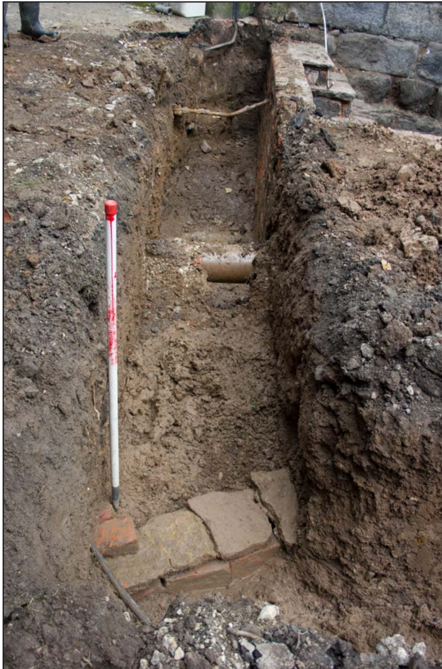
Plate 07: Trench 3 showing location of stone-capped brick culvert at St. Mary's Church, Bosley, Macclesfield - from the south - scale 1m
