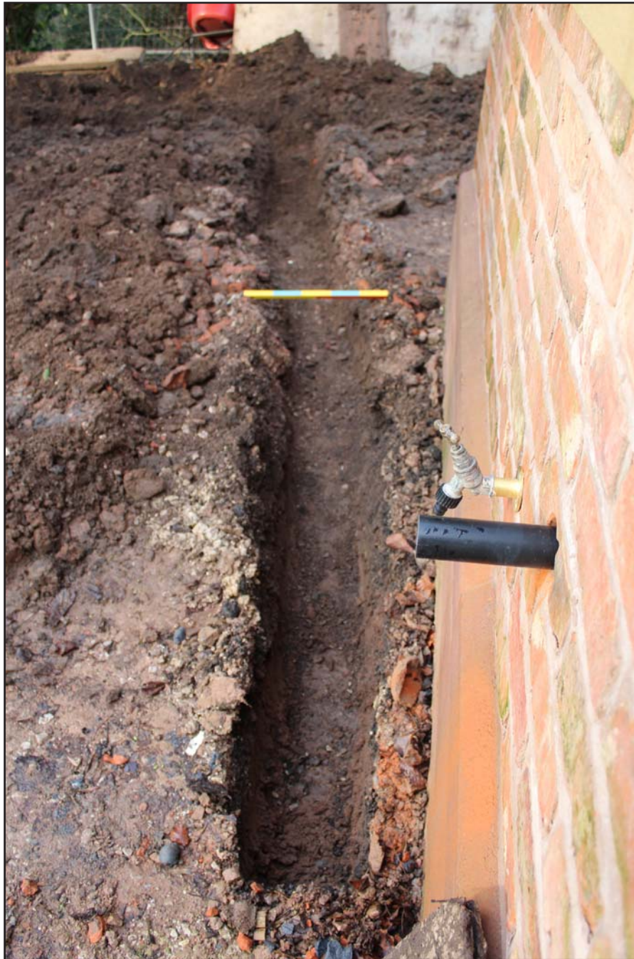
Plate 19: Small drain post excavation at St. Mary's Church, Bosley, Macclesfield - from the east - 0.50m scale
