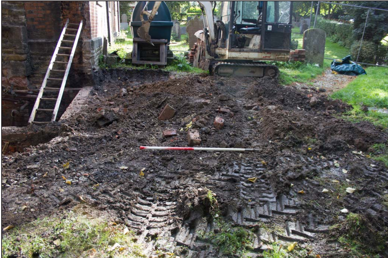
Plate 01: Pre excavation shot of foundation trench area at St. Mary's Church, Bosley, Macclesfield - from the west - scale 1m
