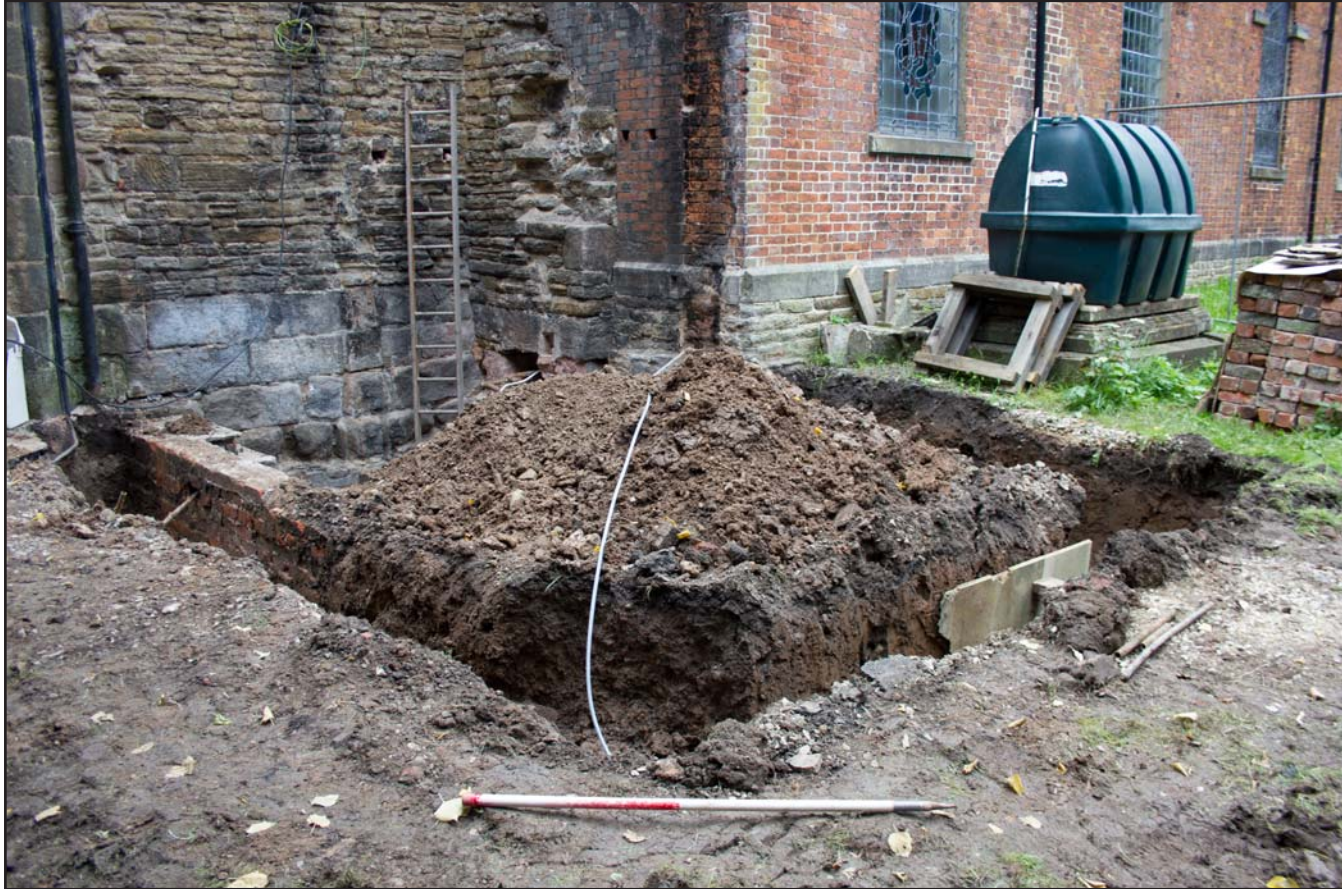
Plate 14: Post excavation shot of foundation trench area at St. Mary's Church, Bosley, Macclesfield - from the southwest - scale 1m
