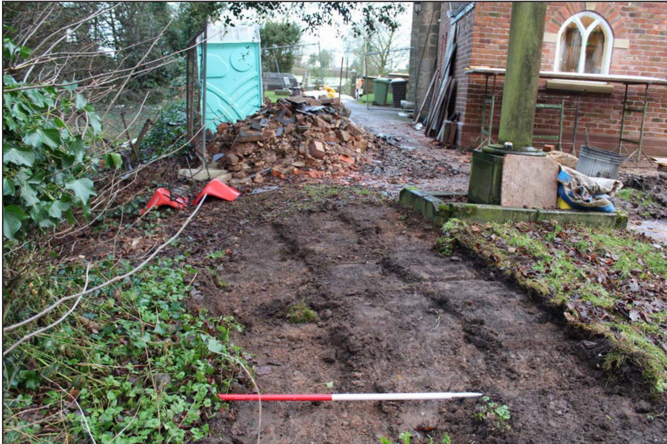
Plate 16: Pre excavation shot of area for sump and drainage trenches at St. Mary's Church, Bosley, Macclesfield - from the south - 1m scale
