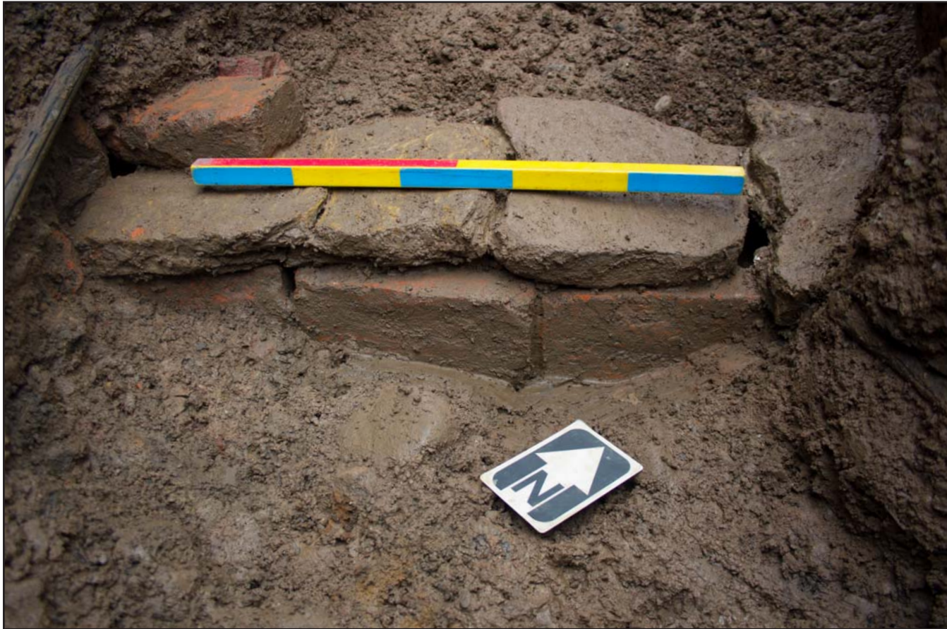
Plate 10: Profile of stone-capped brick culvert at St. Mary's Church, Bosley, Macclesfield - from the southeast - scale 0.50m
