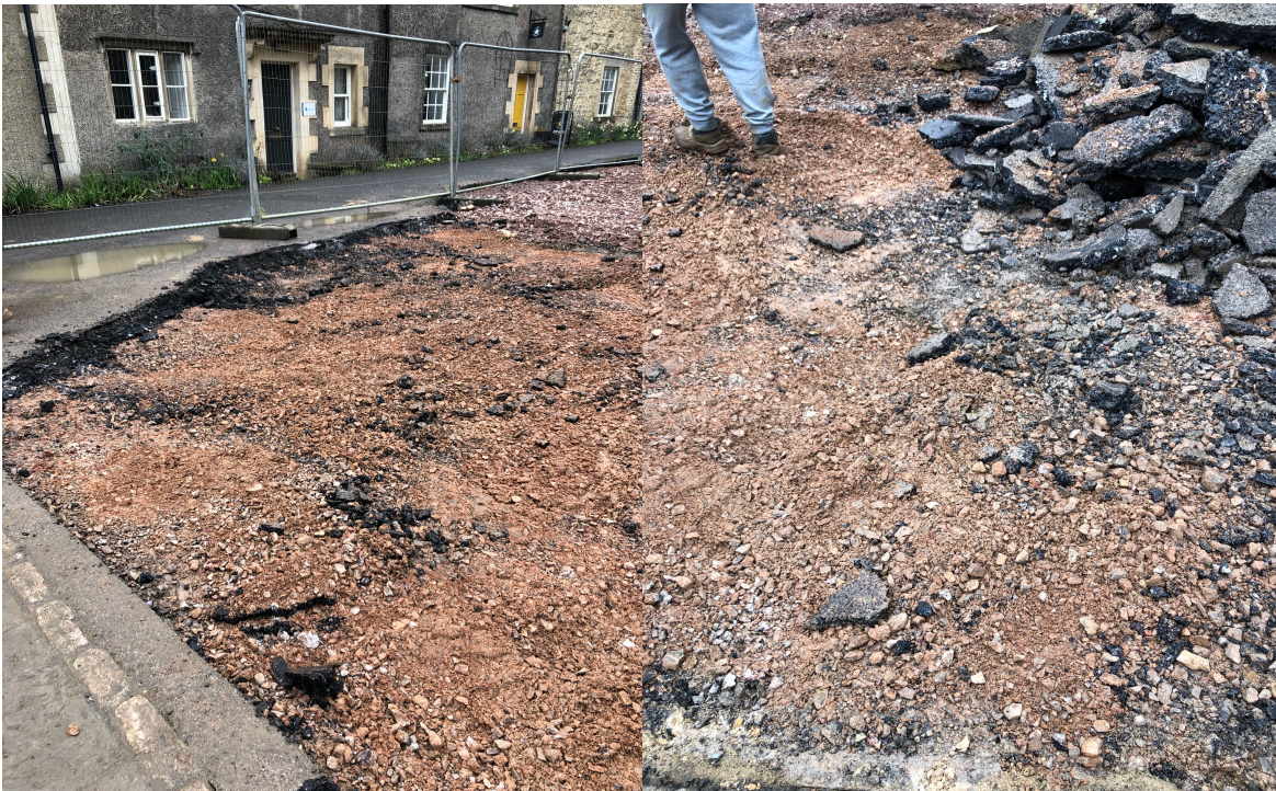
Plates 8 and 9: Removal of modern tarmac and screed underfill in advance of York paving.
