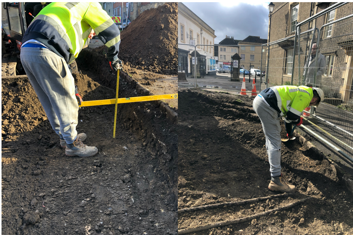
Plate 3 (left) leveling to ensure accurate depth; Plate 4 (right) gas services identified during excavation
