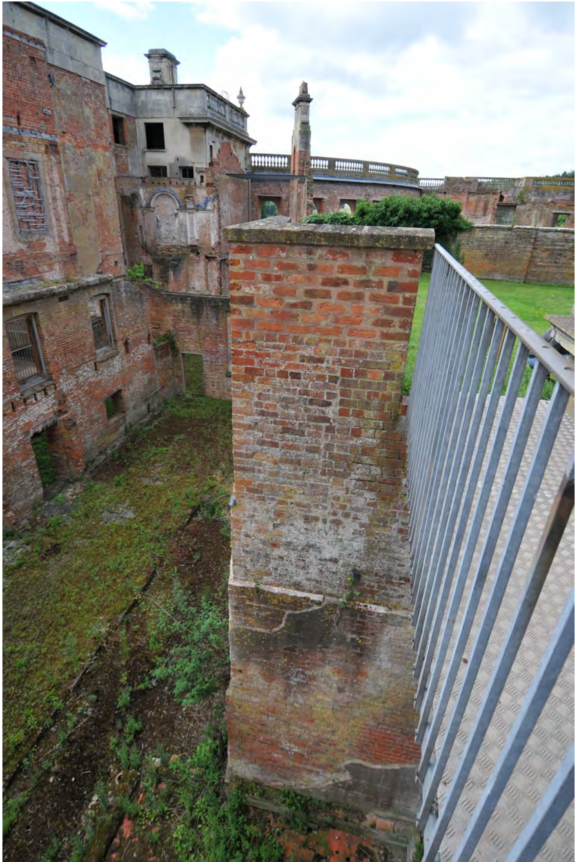
Retaining wall and sunken service yard of Witley Court immediately to east of fire exit ramp
