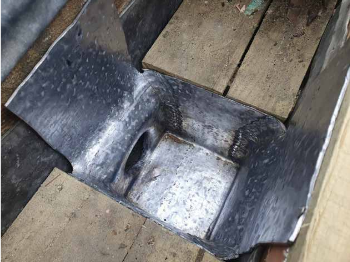
One of the new lead sumps installed, with outlet through the parapet.
