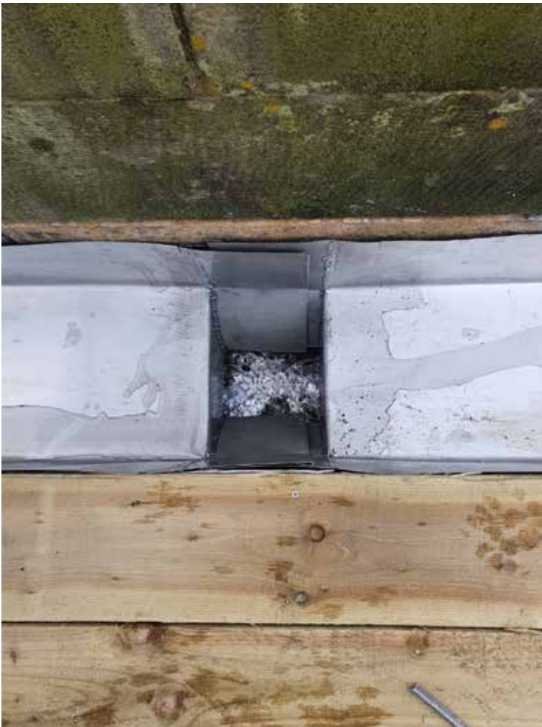
The stainless steel gutter and sump.
