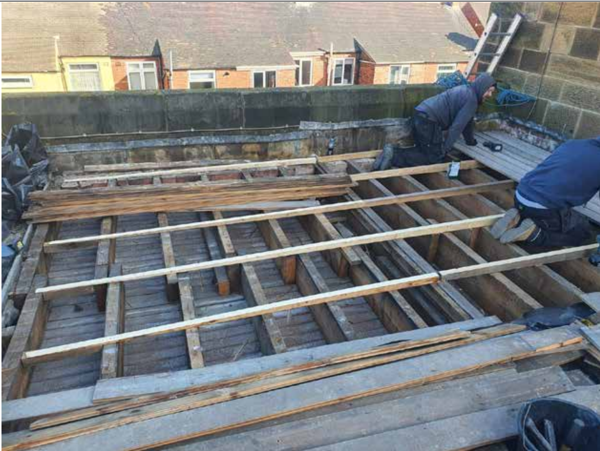
With the lead stripped the boarding under was lifted and relaid on new furrings to a better pitch (3 degrees).
