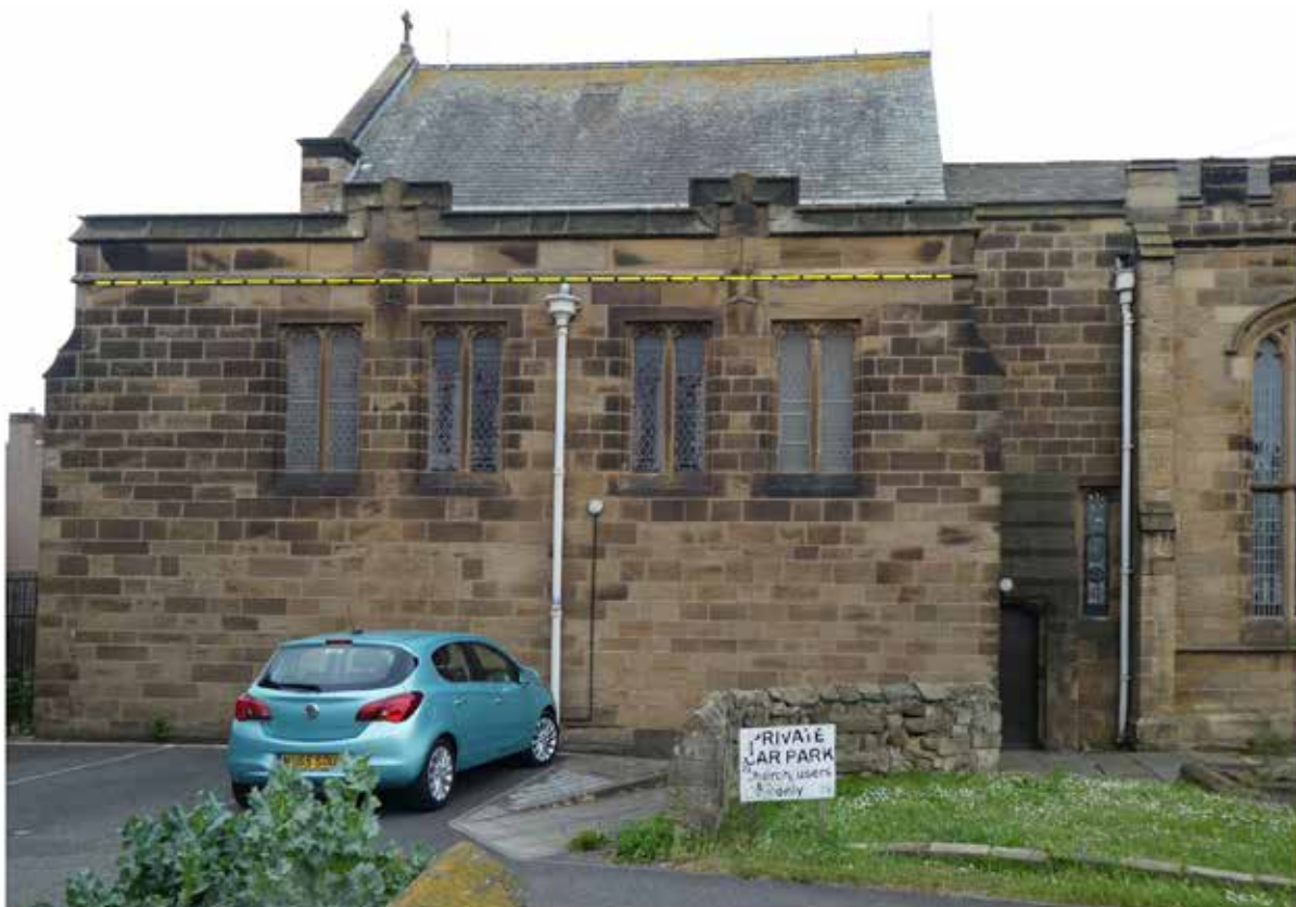
South elevation of Lady Chapel. The yellow dotted line indicates the roofgutter line behind the parapet.
