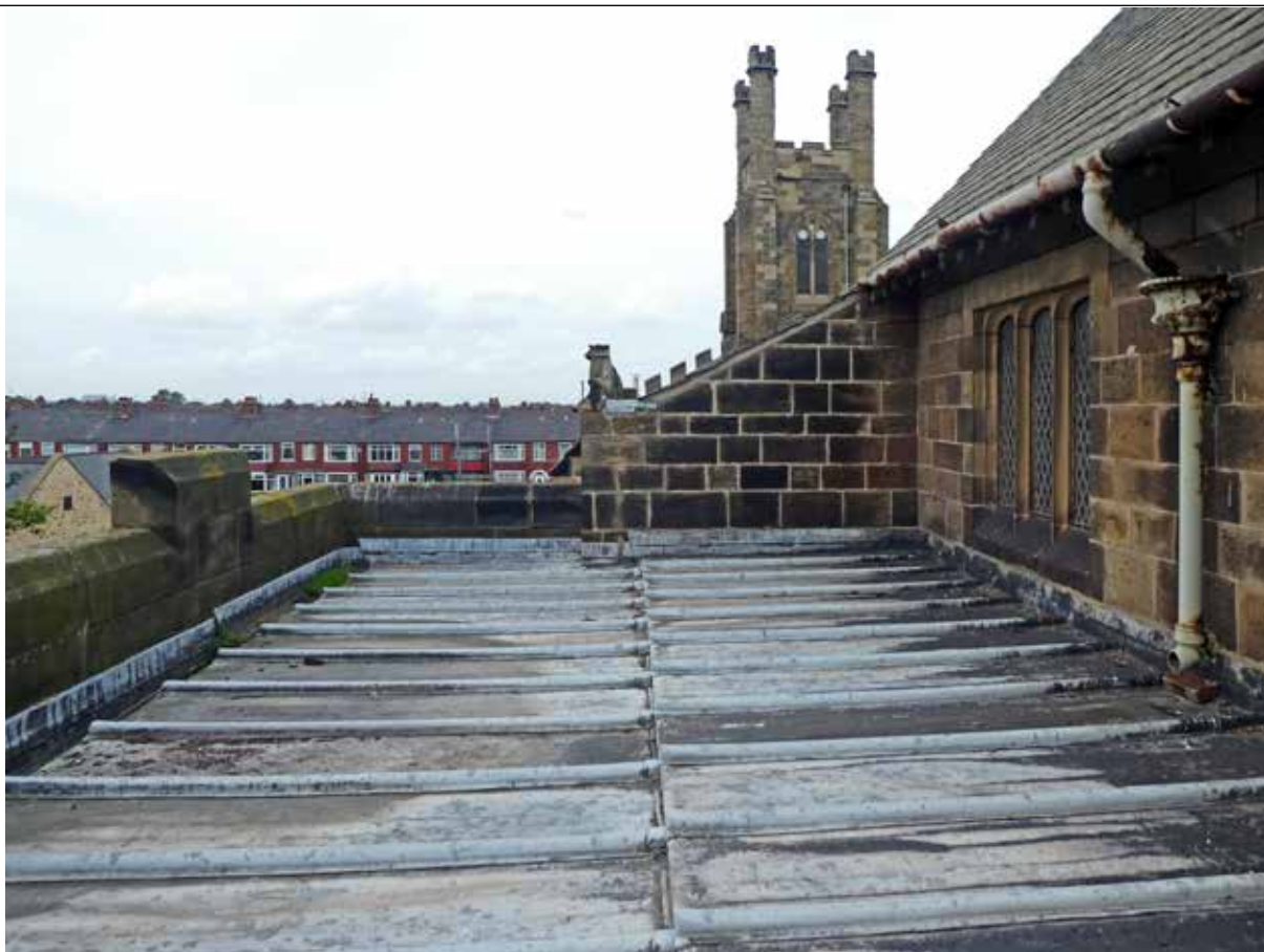
The existing lead roof on north side of Chancel (looking west). The limited length of lead bays required a step to be formed resulting a very shallow pitch resulting in ponding of water, indicated by dark patches on the lower sections of roof. This photo was taken in 2019 before the cast iron gutter was taken down due to concerns over its condition and fixing.
