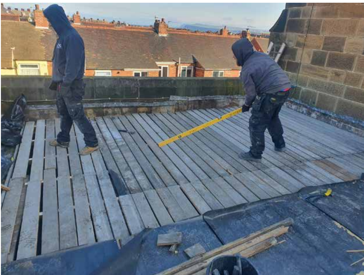
The existing boarding relaid, ready to receive the new roof build up.
