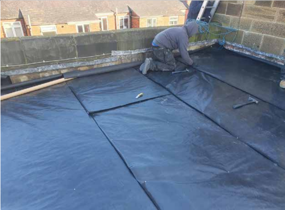
Installation of the new breather membrane which sits under the insulation layer.
