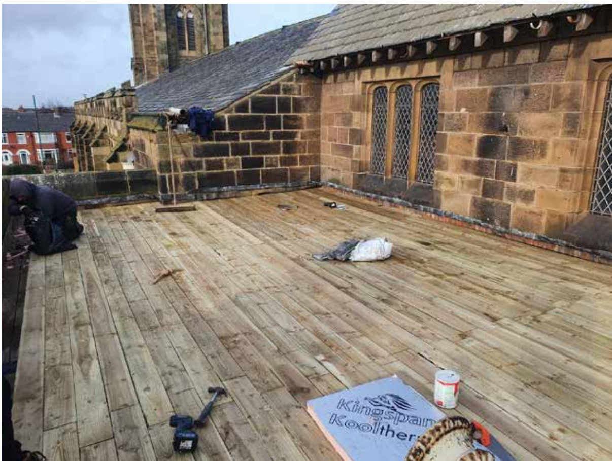
A top layer of boarding supports a Permo Sec membrane and stainless steel finish.
