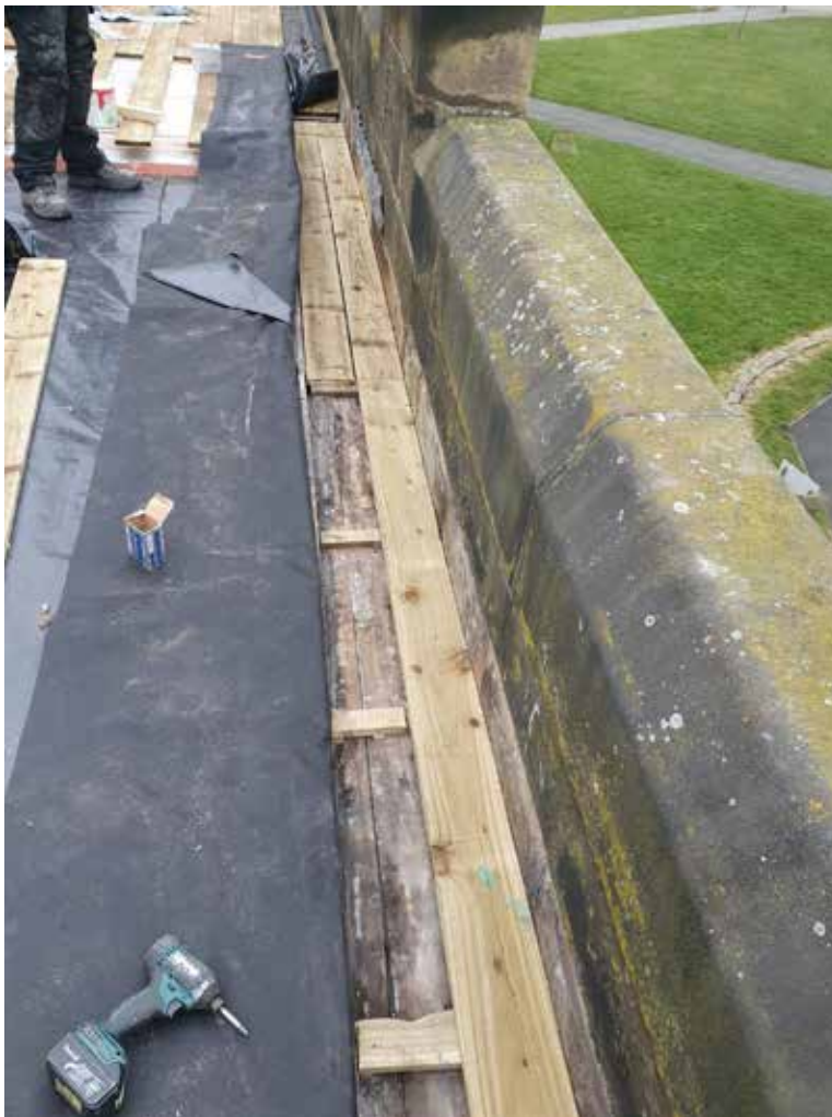
Some of the existing boards under the parapet gutter were affected by rot. This shows the installation of new gutter boards.
