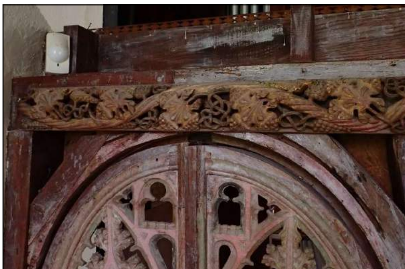
Detail of east face cornice, showing ornate running ornament, originally from the west face. The white bloom is a degraded wax coating obscuring the paint.
