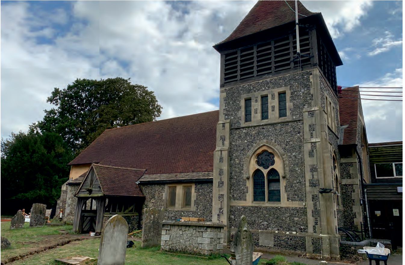
Plate 1. General of the northern side of St Mary's Church, Main Road, Longfield showing the nineteenth century additions (tower, nave and north aisle west end) added onto the earlier medieval nave, north aisle, north porch and chancel.
