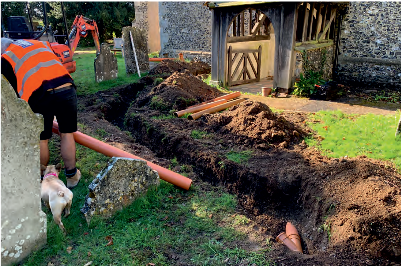
Plate 4. General view looking southeast showing drainage trench DT 3 in relation to the north porch.
