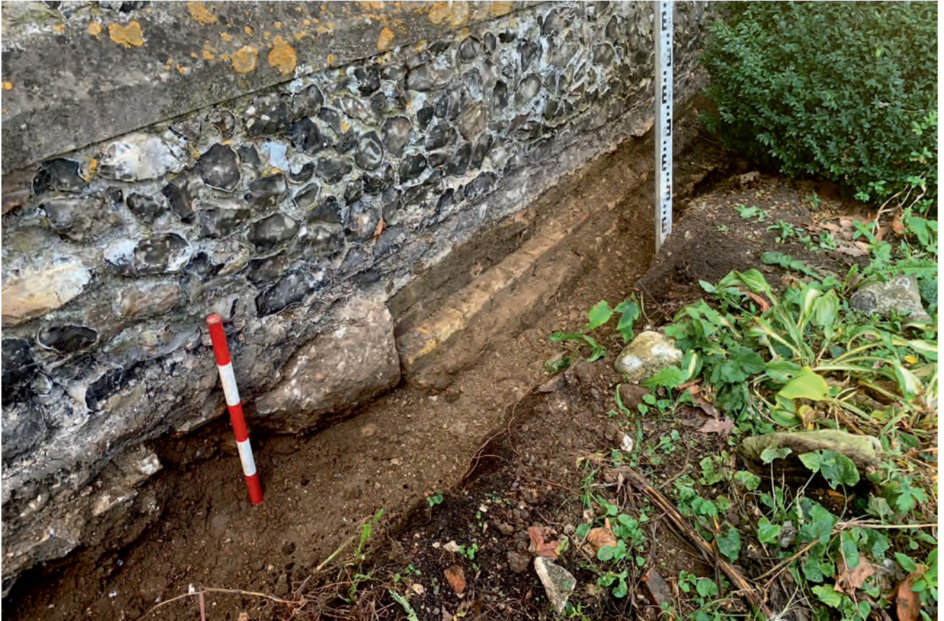
Plate 5. View looking southwest along the line of drainage trench DT1 extending along the base of the north wall of the north aisle showing corner stone to medieval foundation abutted by brick foundation of later west tower and nave extension.
