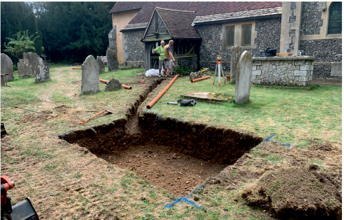
Plate 2. General view looking southeast across Soakaway position S1 and showing drainage trench DT1 within the northern portion of the churchyard.
