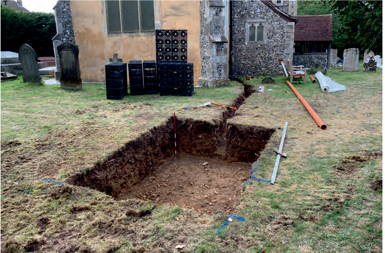
Plate 3. General view looking east showing soakaway position S2 and drainage trench DT2 in relation to the east end of the chancel.
