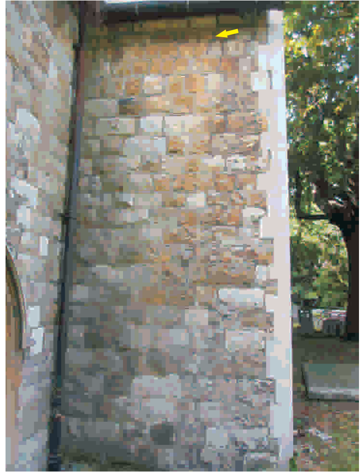
Photograph 6. View of the north-eastern elevation of the North Porch with what could be a small crack (arrowed)
