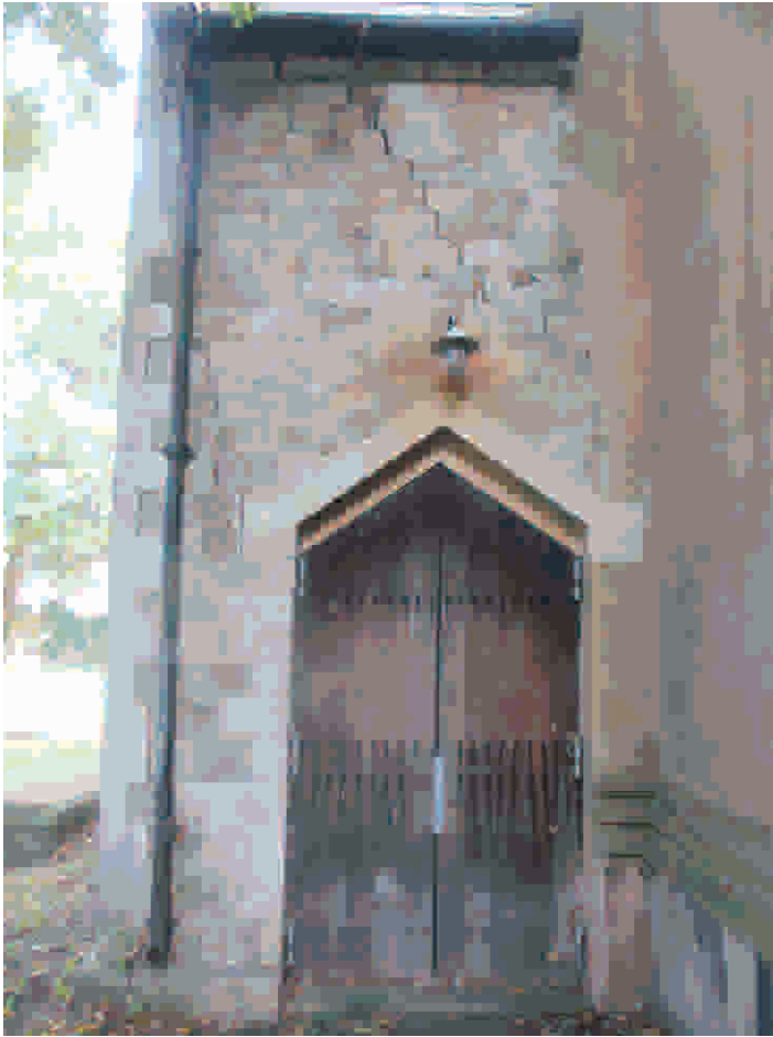
Photograph 5. View of the south-western elevation of the North Porch showing the cracking angled upwards to the west
