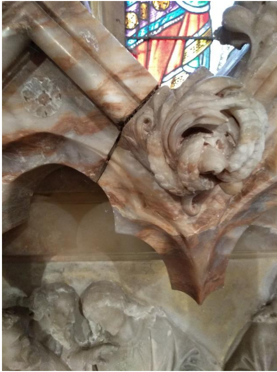
Figure 15: Open joint to the canopy
