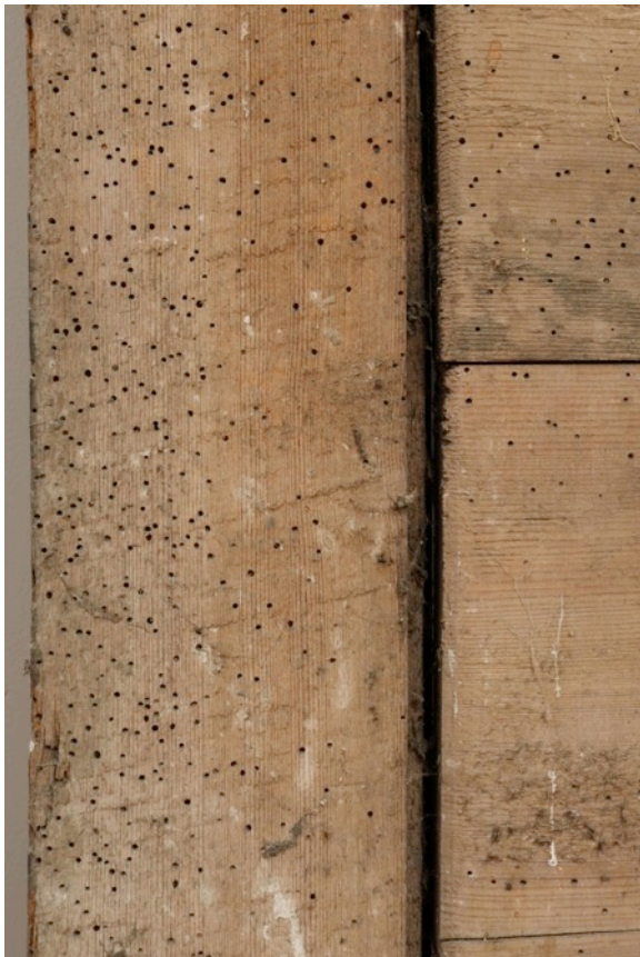
Plate 4 Detail of woodworm infestation on panel and frame
