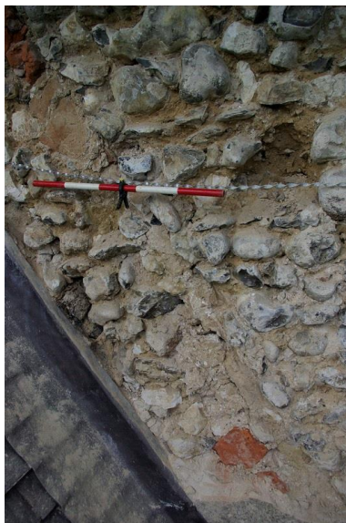
Plate 52: Nave former gable scar [15], N side, timber visible (left/central) looking W, 0.5m scale
