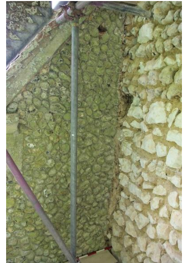
Plate 27: N side of tower abutting former nave wall, with Victorian flint wall, looking ESE. 0.5m scale
