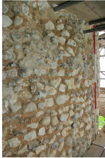
Plate 32: W side, central stage [34], infilled patch, [71] (top left), window [17] to left of 2m scale, looking S
