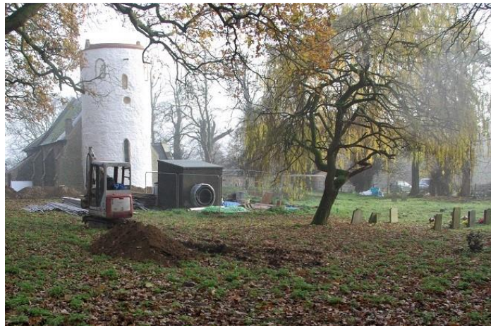
Plate 21: Trench 65, for reinterment of human remains in NW churchyard, looking ESE (contractor's site hut in place)
