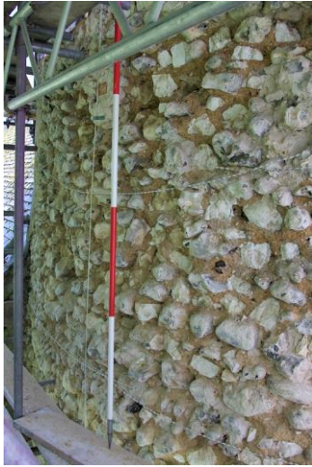
Plate 31: N side, central stage [34], infilled patch, [66] (top left, brick visible), looking ESE, 2m scale
