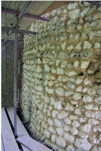
Plate 25: N side, lower stage [33], chalk courses, window [30] visible (bottom left), looking E, 2m scale
