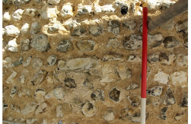
Plate 44: Blocked putlog hole ([8]), north of window [11], flint 'framing' at top and lighter mortar within, looking E 0.5m scale (red)
