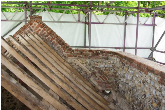
Plate 50: Internal view of area of blocked pentagonal opening, and gable roof rafters exposed, looking N
