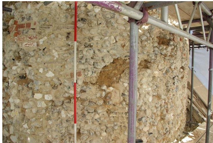
Plate 34: S side, central stage, wall exposed with on-going repairs in progress, looking E, 2m scale
