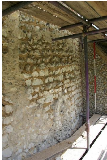
Plate 26: S side, lower stage [33], with [34] above, window [31] visible, looking E, 2m scale
