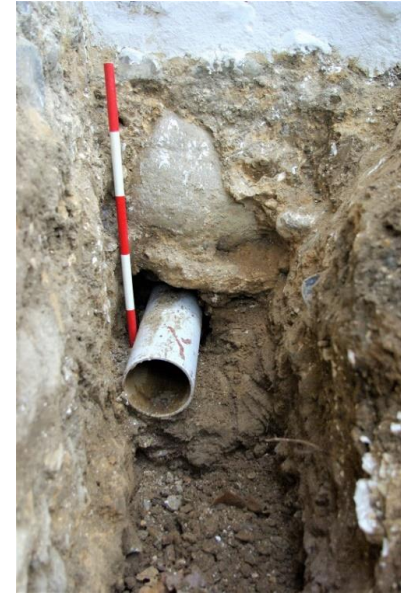
Plate 20: Trench 60, base of tower N wall and new downpipe looking S, 0.5m scale
