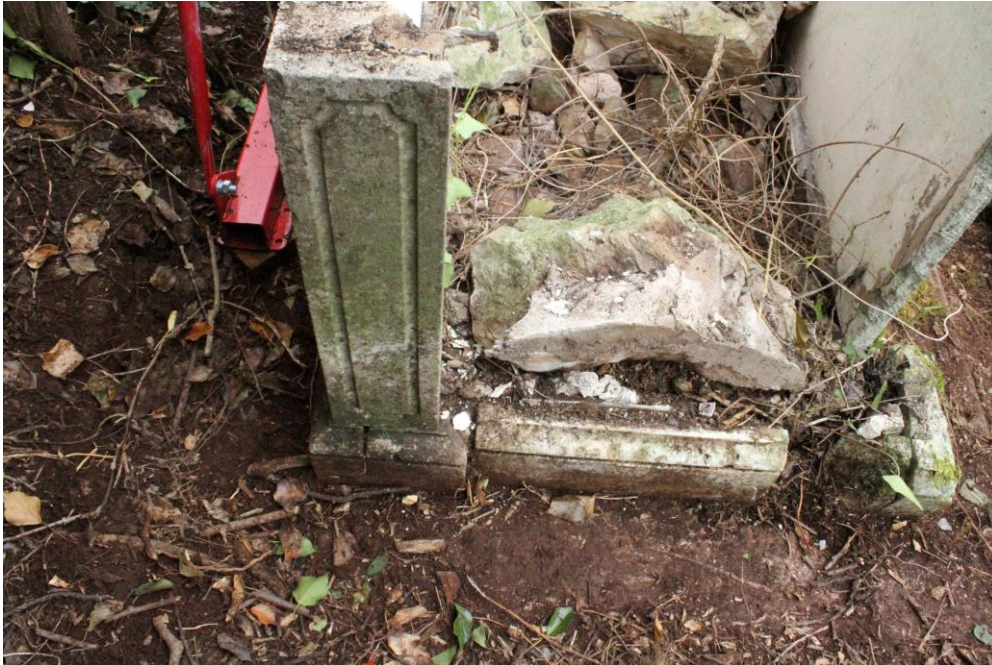
9 and 10. Right; poor quality internal support system to the Hunt tomb; below, moss and open joints in the plinth and base
