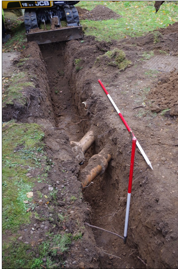
Photo 7. Detail of old drains and inspection chamber outside north door, looking W.
