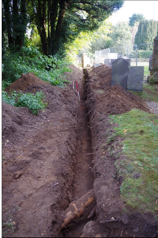
Photo 3. View of excavated service trench on line of path, looking ENE towards Main Street.
