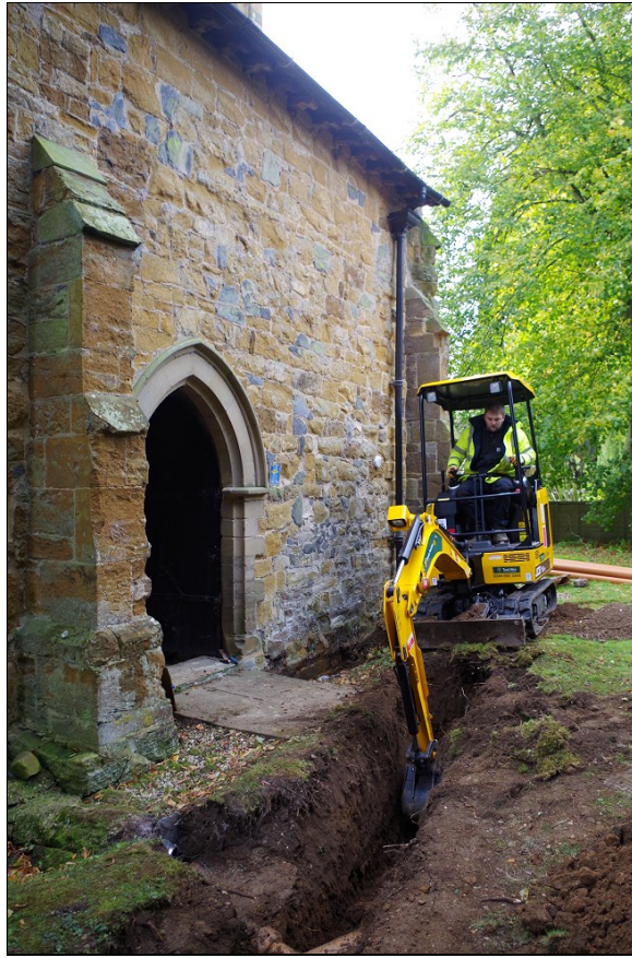
Photo 5. Excavation of service trench adjacent to north door of church, looking WSW.
