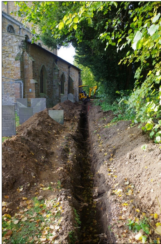
Photo 4. View of excavated service trench on line of path, looking WSW towards N door.
