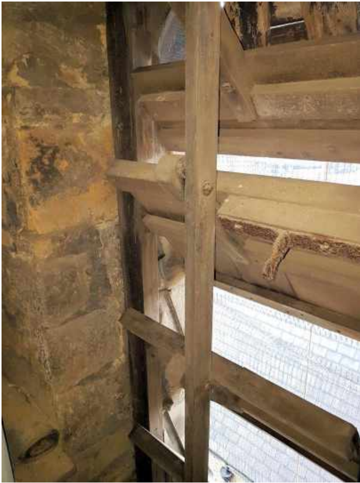
Louvres operating but impeded by netting
