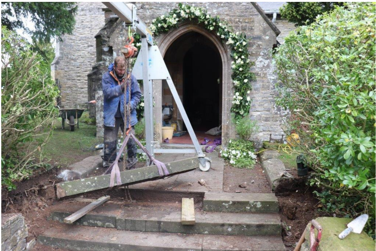
Plate 10: Lifting the steps using specialist equipment, following removal of adjacent church walls. View northwest
