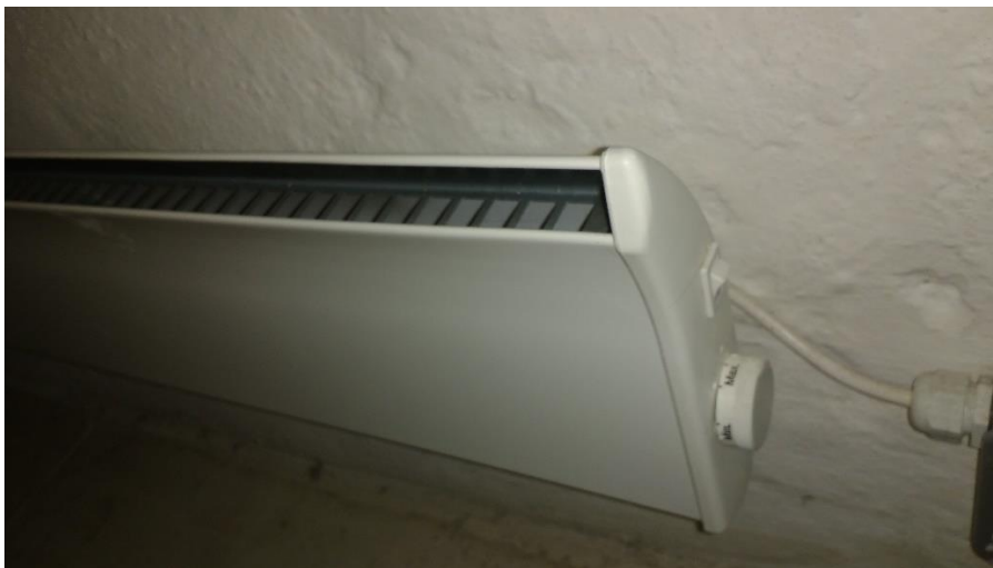
Panel heaters (4, Norel, 1kW each) are fitted in the choir area.
