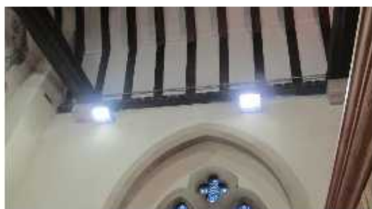
Lighting in the vestry/kitchen area
