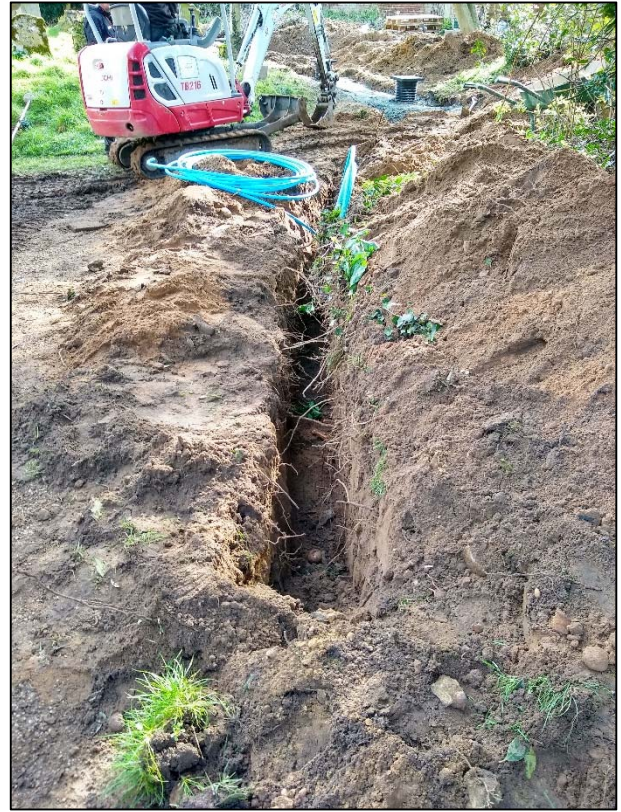
Plate 5. Water pipe trench, north side of the path. Looking east towards the trench arch drain
