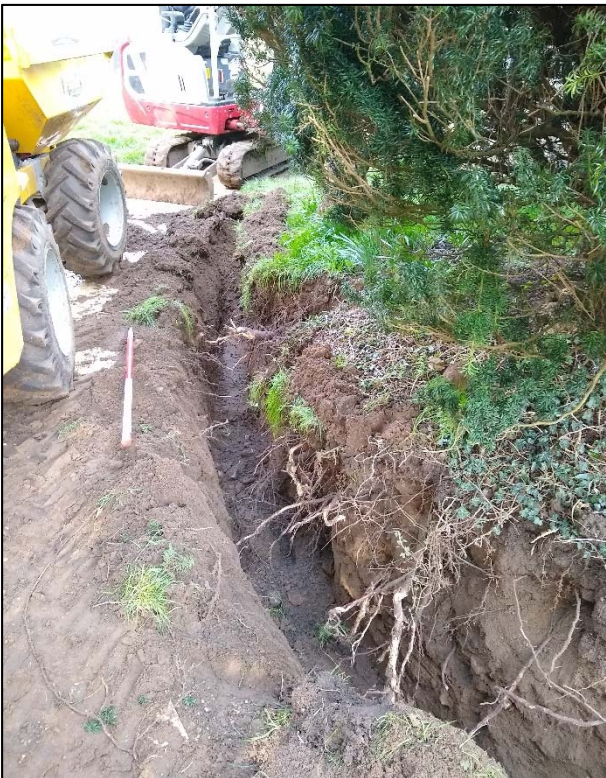
Plate 6. Water pipe trench, north side of the path. Looking north, 1m scale
