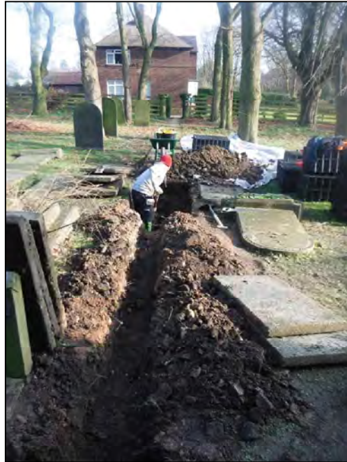
Plate 1. Working shot showing excavated trench and excavation of the soakaway, facing east
