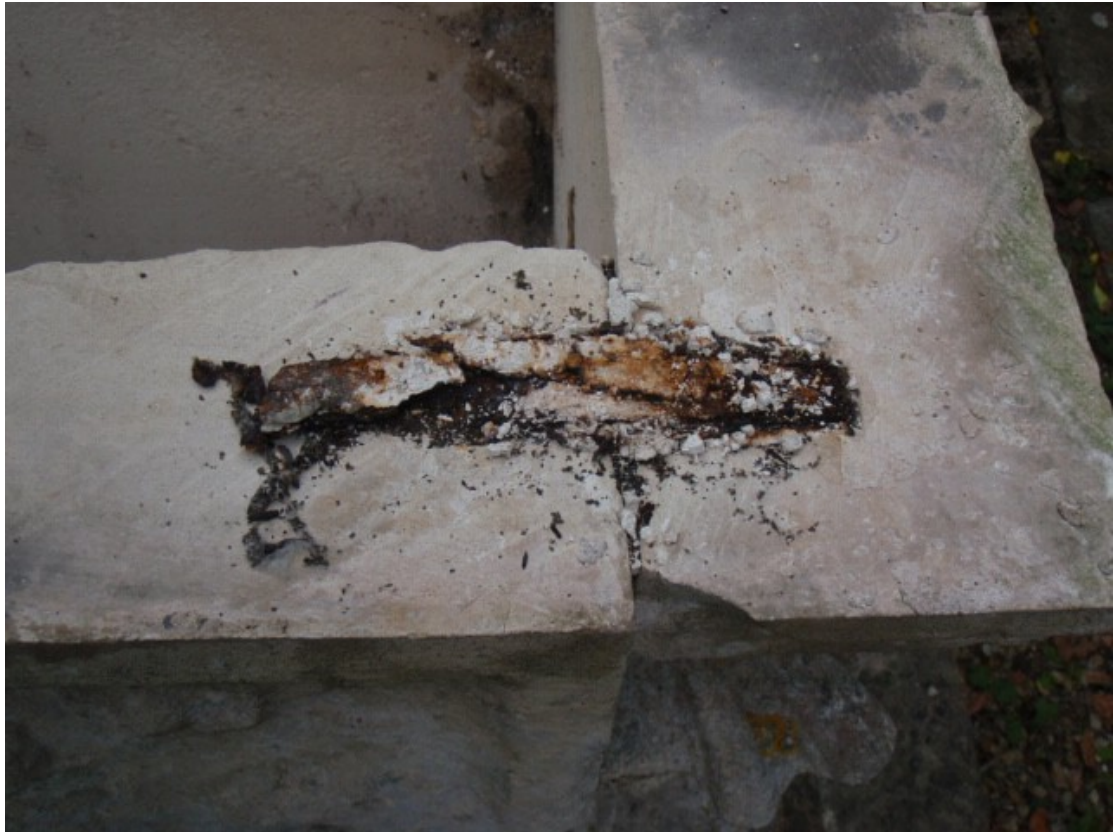
A rusting iron cramp.
