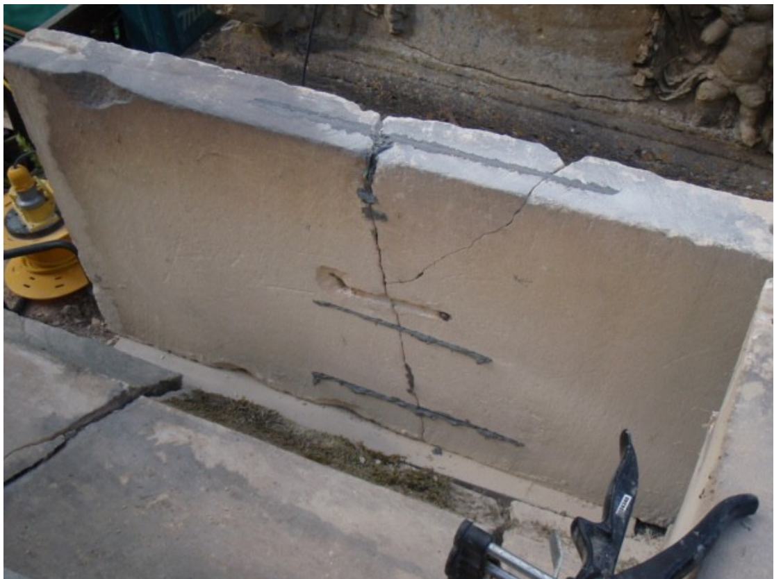
The broken panel was then reinforced using stainless steel bars set into slots.
