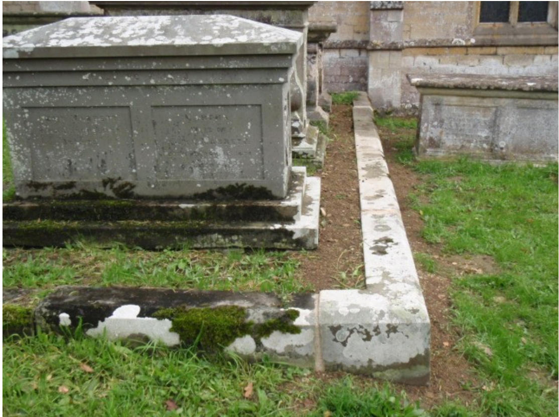
The works completed, from the N, with joints pointed and soil reinstated.
