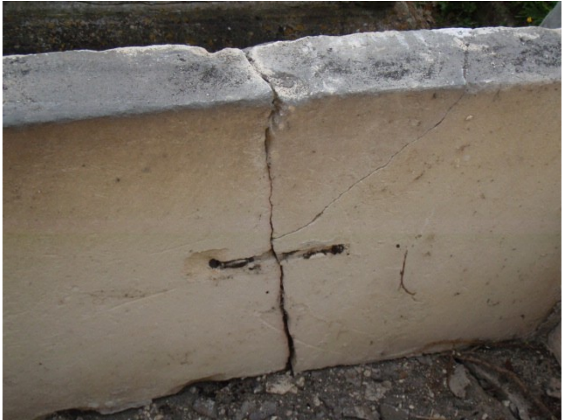
The north side panel, showing an iron cramp from a previous repair.
