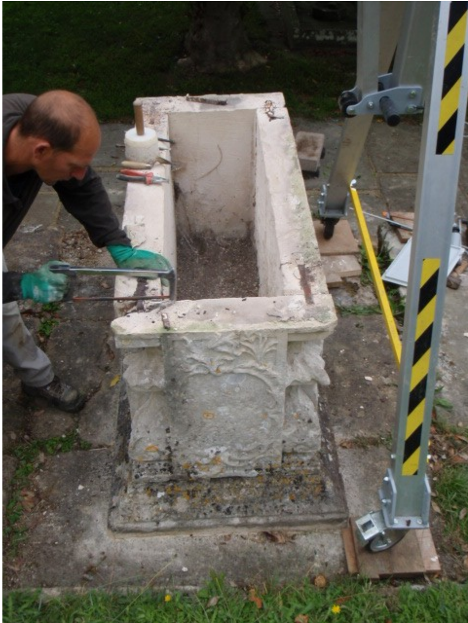
The top was removed using a lifting gantry, and the rusted iron cramps taken out.
