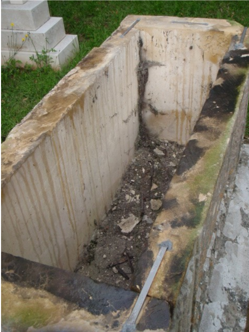
The lid was removed, and the iron cramps replaced by stainless steel ones.
