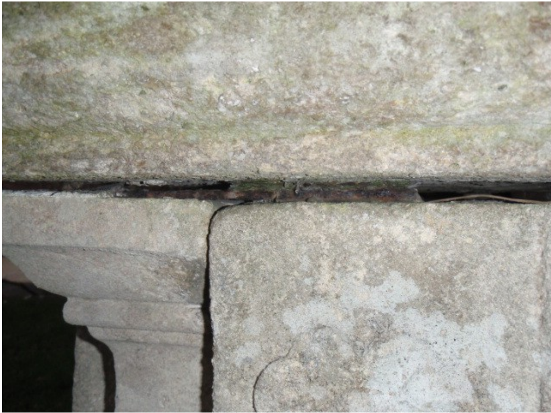
A rusting iron cramp lifting the lid at the south-west corner.
