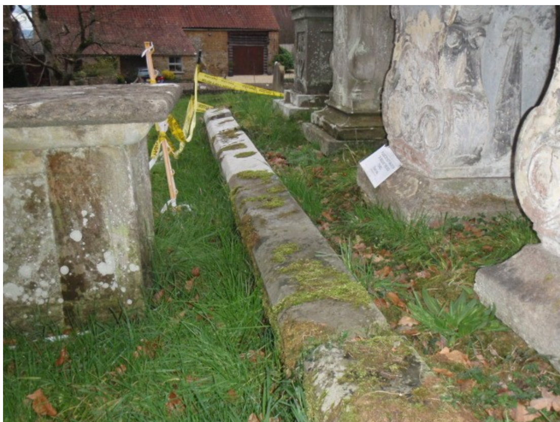
The plinth stone is subsiding towards the west.
