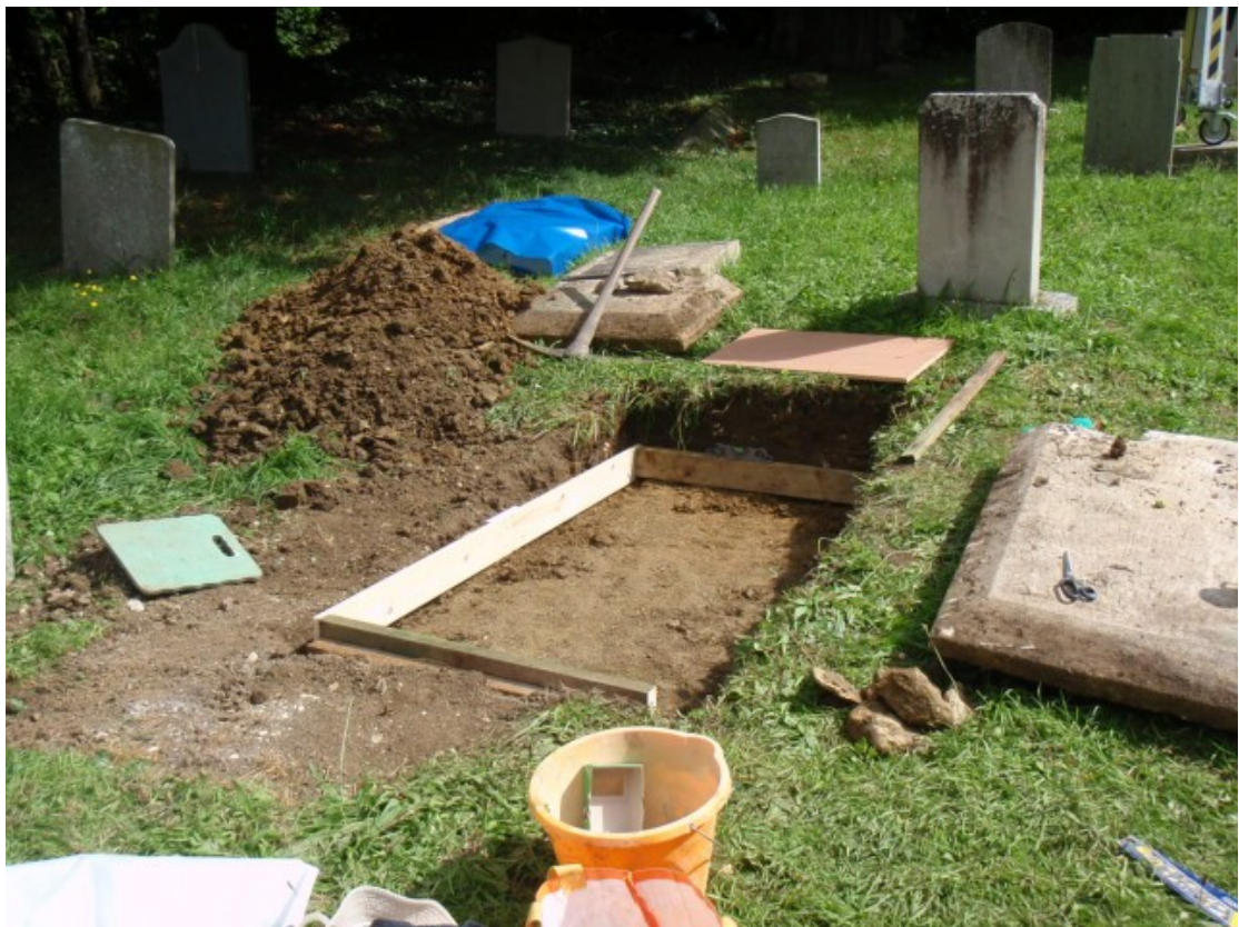
After lifting out the plinth stone, the area was prepared for a limecrete foundation.
