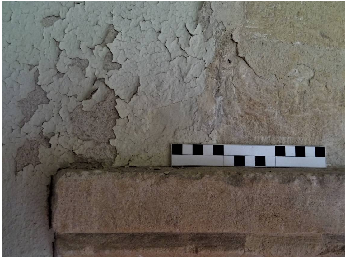
Plate 8. Flaking lime-wash from around the upper section of the door casement
