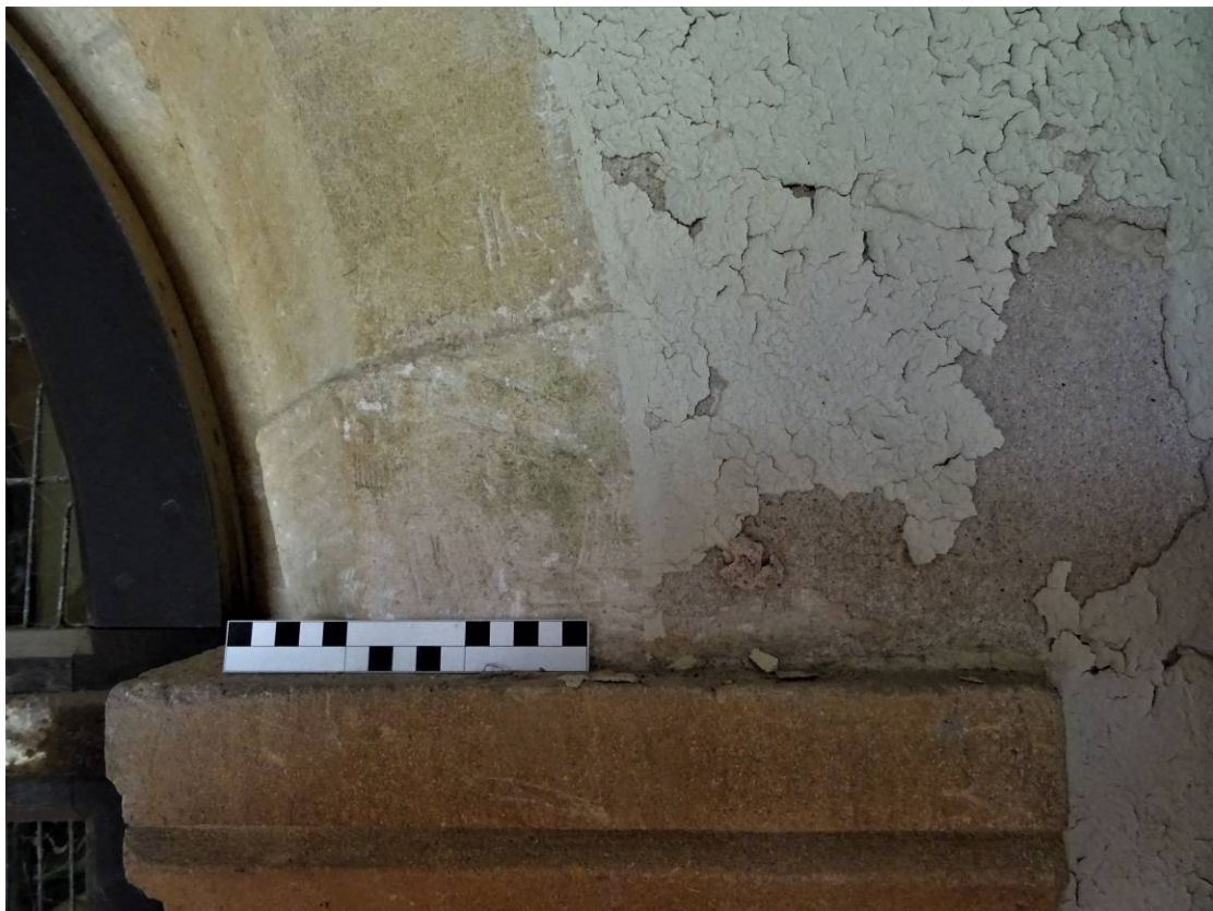
Plate 9. Flaking lime-wash from around the eastern upper section of the door casement
