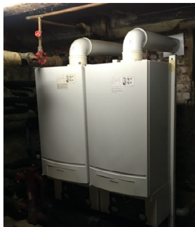
Photograph 3: Gas Combination Boilers
