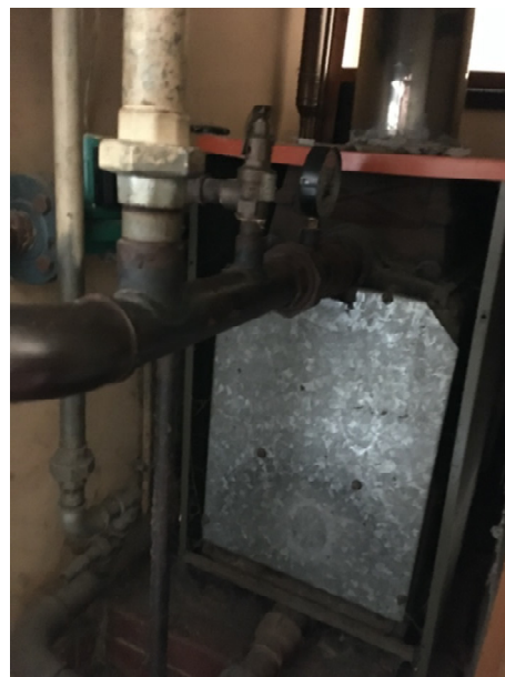
Photograph 3: Immersion Heater with Pipework
