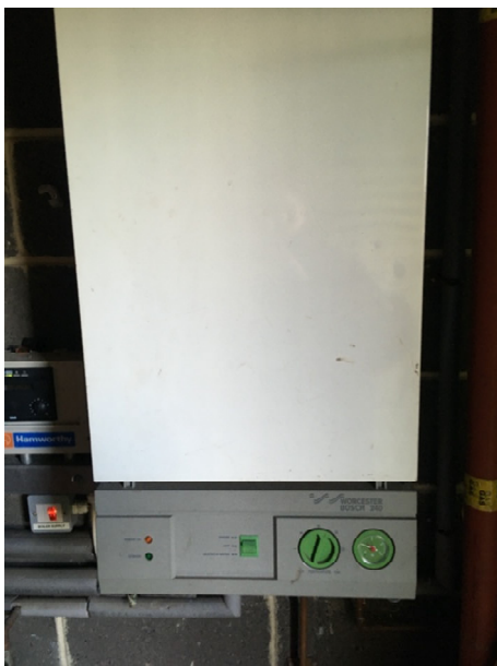
Photograph 2: Gas Combination Boiler
