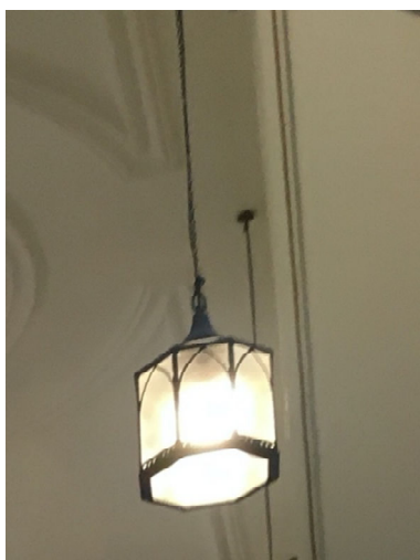
Photograph 7: LED Hanging Lamps
