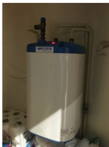
Photograph 5: Electric Water Heater
