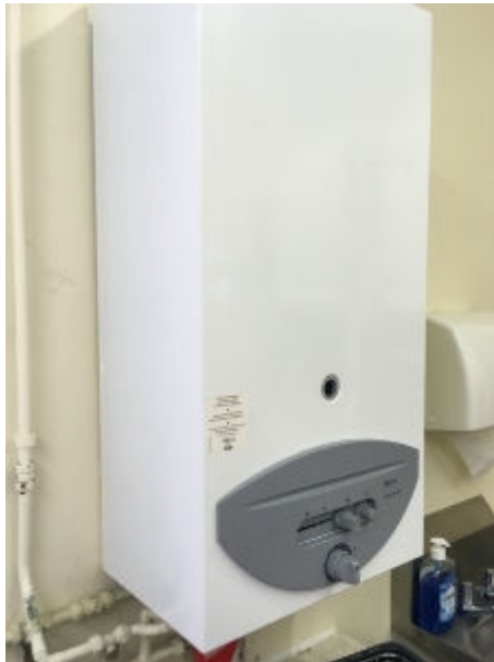
Photograph 1: Gas Multipoint Boiler
