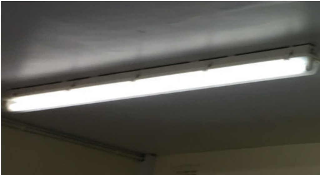
Photograph 6: T8 Fluorescent Tubes
