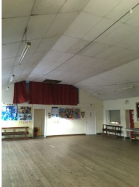
Photograph 5: T8 Fluorescent Tubes
