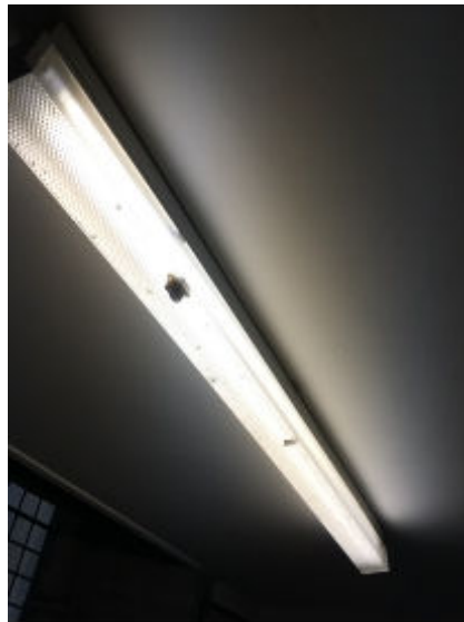
Photograph 7: T8 Fluorescent Tubes
