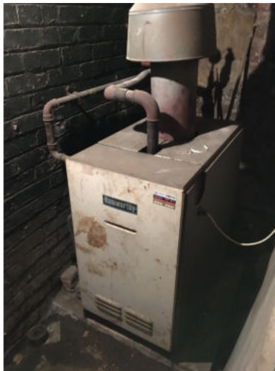
Photograph 2: Gas Fired Boiler
