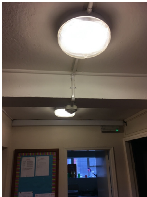
Photograph 11: Compact Fluorescent Lights
