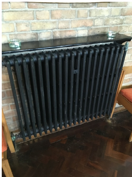
Photograph 5: Church Hall Radiators
