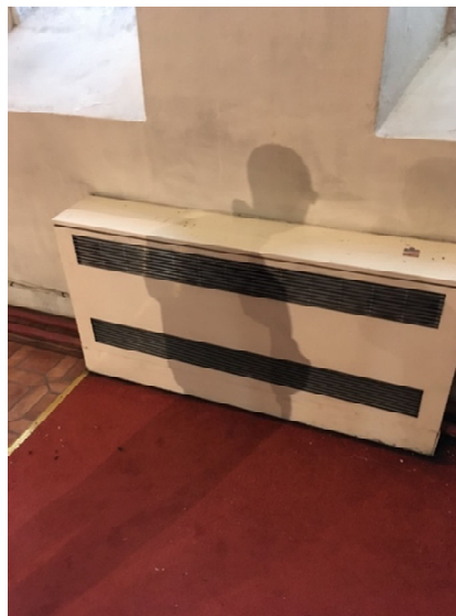
Photograph 4: Church Hall Radiators
