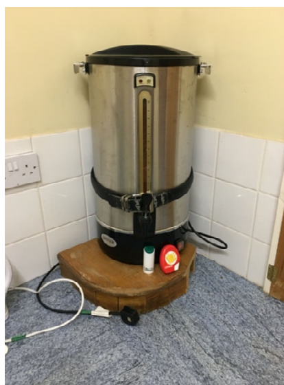
Photograph 5: Electric Water Heater
