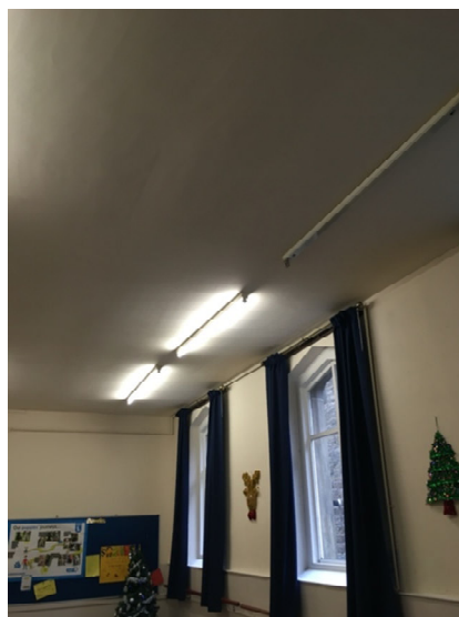
Photograph 5: T8 Fluorescent Tubes
