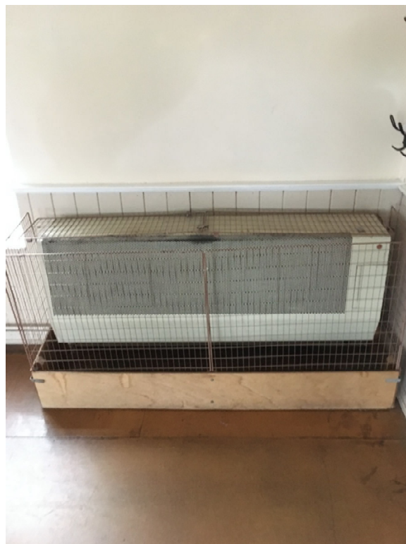
Photograph 2: Church Heat Emitter
