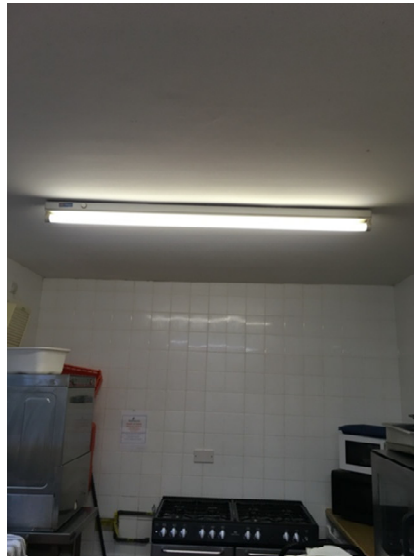
Photograph 6: T12 Fluorescent Tubes
