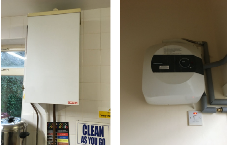
Photographs 3 & 4: Water Heaters
