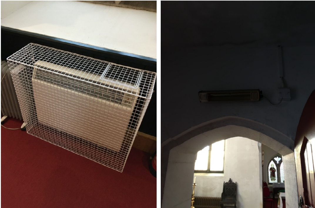
Photographs 3 & 4: Church Heat Emitters
