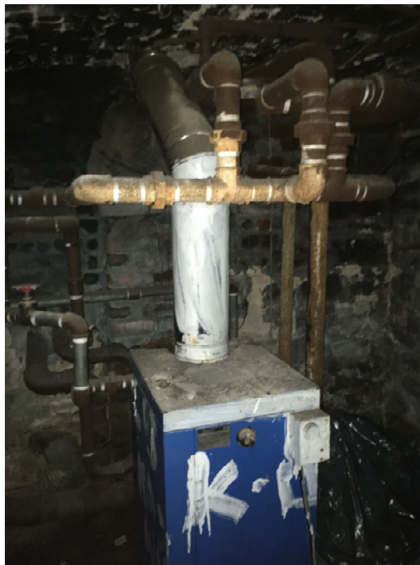
Photograph 2: Church Boiler – Disconnected
