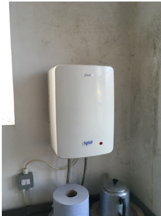
Photograph 5: Omega Water Heater
