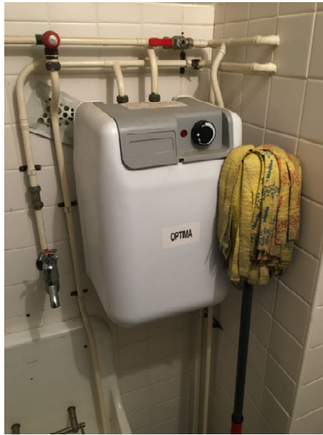
Photograph 6: Electric Water Heater
