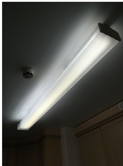
Photograph 12: Twin Fluorescent Tube
