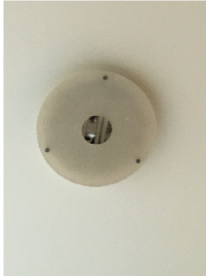
Photograph 13: Twin Fluorescent Spotlights
