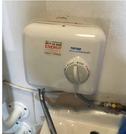
Photograph 6: Electric Point of Use Water Heaters
