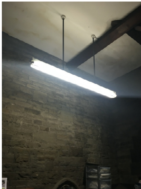
Photograph 12: Twin Fluorescent Tube
