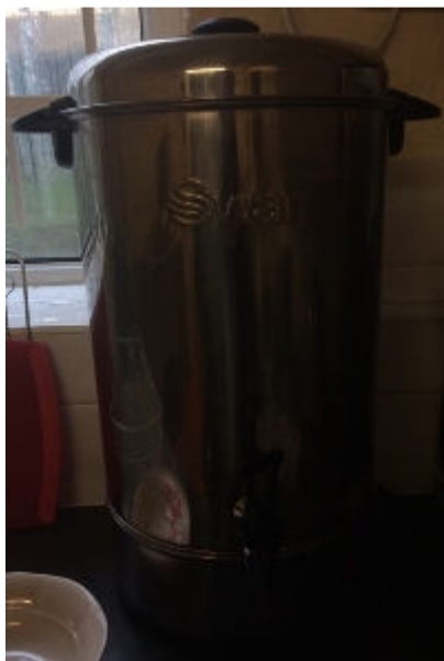
Photograph 9: Electric Point-of-Use Water Heater
