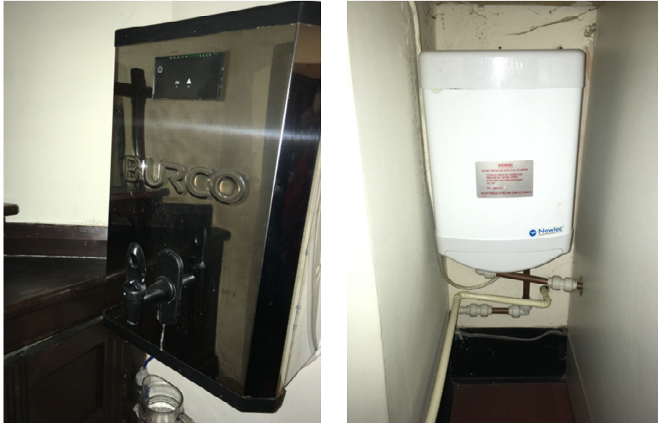
Photographs 7 & 8: Water Heaters
