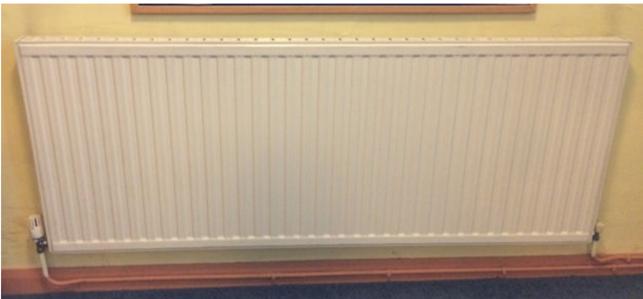
Photographs 6&7: Church Heat Emitters
