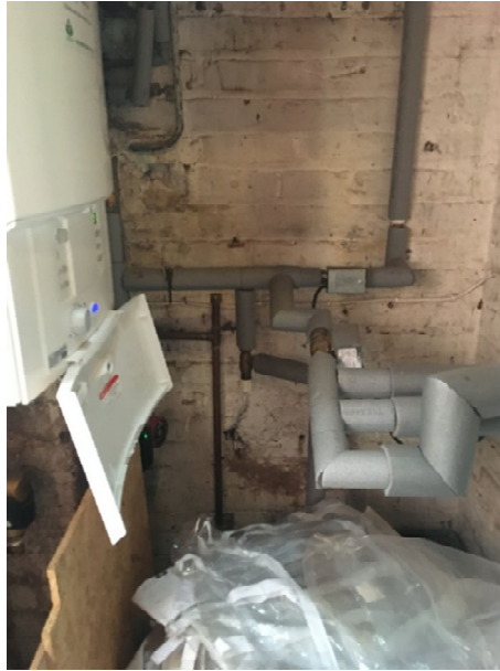
Photograph 3: Heating System Pipework
