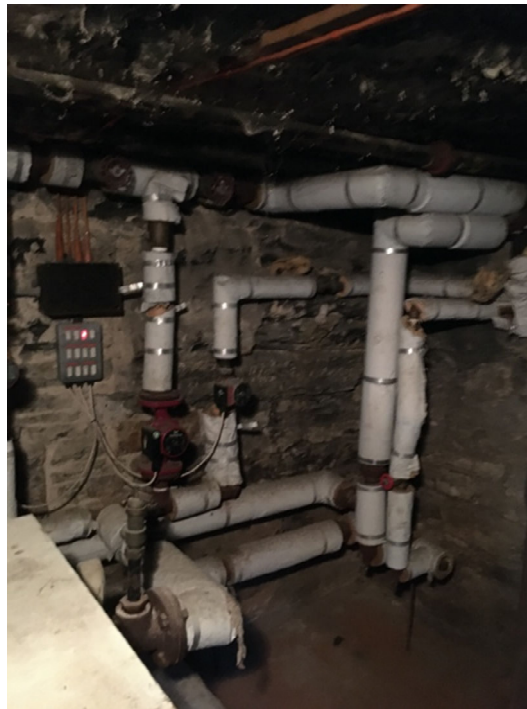
Photograph 3: Heating System Pipework
