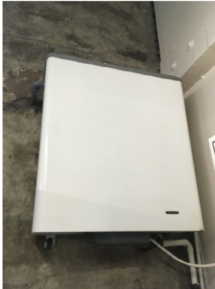
Photograph 5: Electric Water Heater
