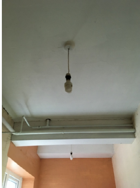
Photograph 11: Fluorescent Pendant Lamps
