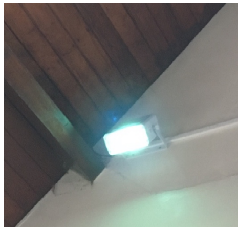
Photograph 8: Metal Halide Floodlights
