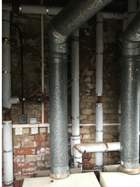
Photograph 3: Heating System Pipework
