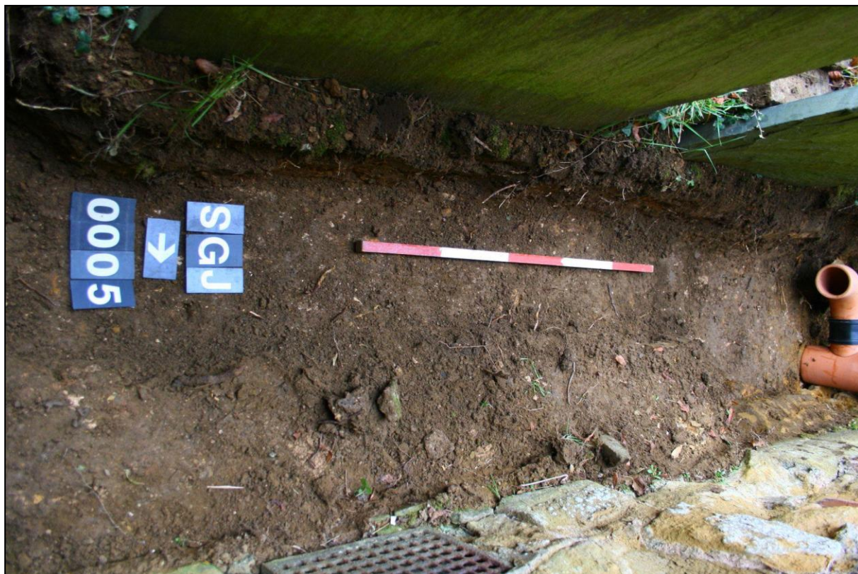
Plate 9: Excavated east-west drain run adjacent to entrance porch showing backfill layer (0005). Scale: 1 x 1m.
