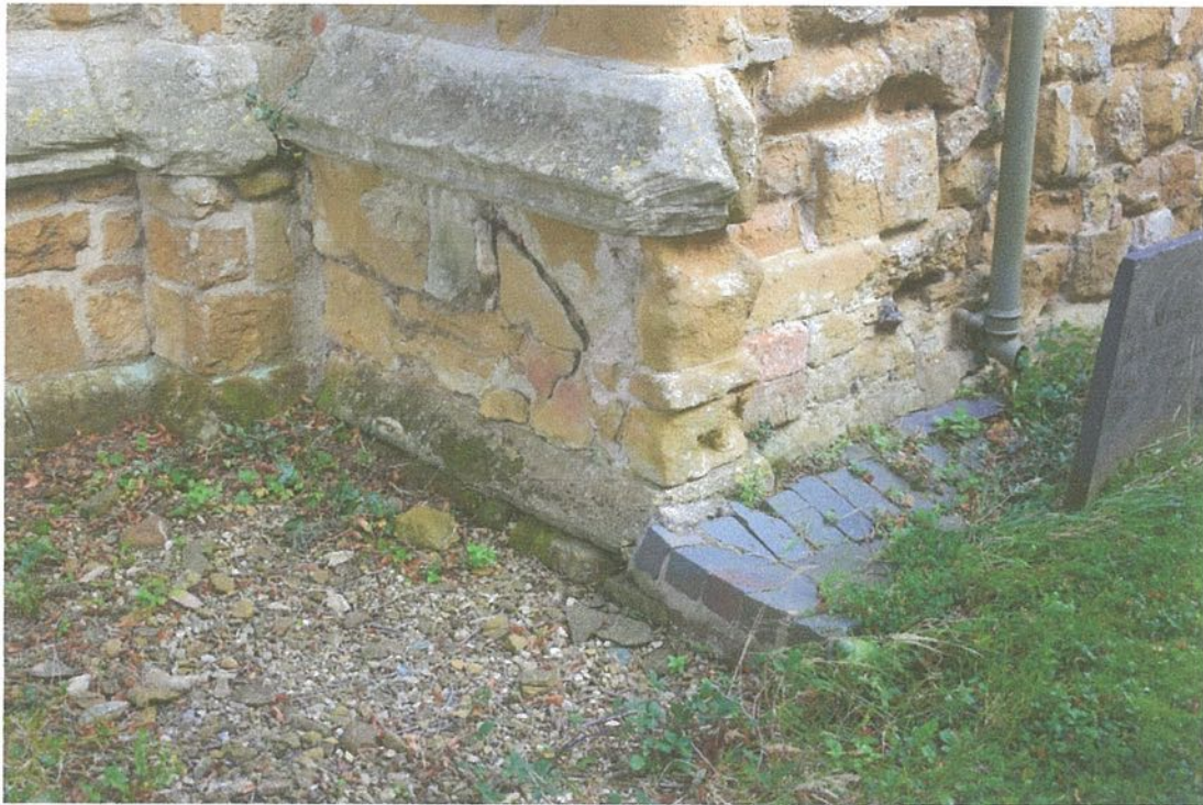
Plate 7: The south-west corner of the nave where the brick drainage channel meets the gravel. The very poor condition of the channel is clear. The limestone weatherings are basically sound. The ironstone visible can be conserved by localised repair, re-pointing and consolidation with mortars as described.
