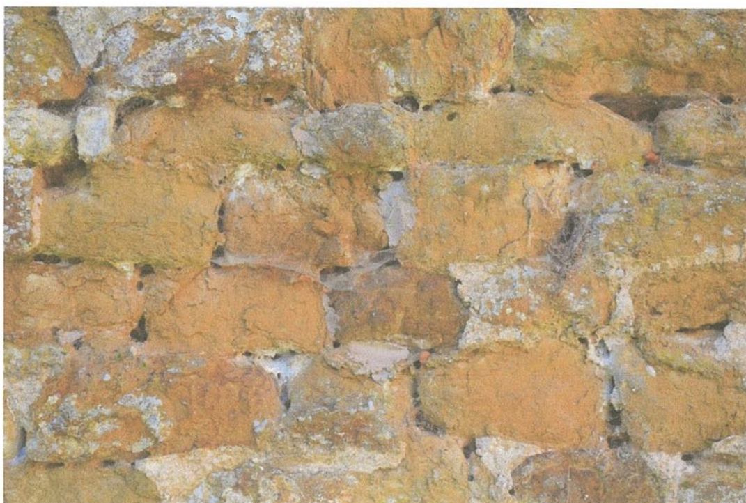
Plate 10 : An area of stonework affected by masonry bees with quite deep and large pockets in the mortar, and lots of old patch repairs in cement. Although in principle it would be nice to be able to accept and accommodate the bees, here they are starting to cause structural problems. The voids here need grouting and filling, and the joints re-pointing in lime mortar. None of the stones visible in this photograph need replacing.
