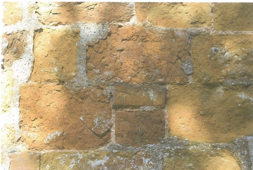
Plate 9 : This area of stonework has not weathered heavily and can just be brushed down and re-pointed in lime mortar.
