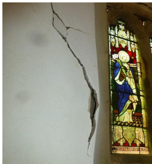
Photograph 8: Gaps associated with plaster at south aspect of chancel
