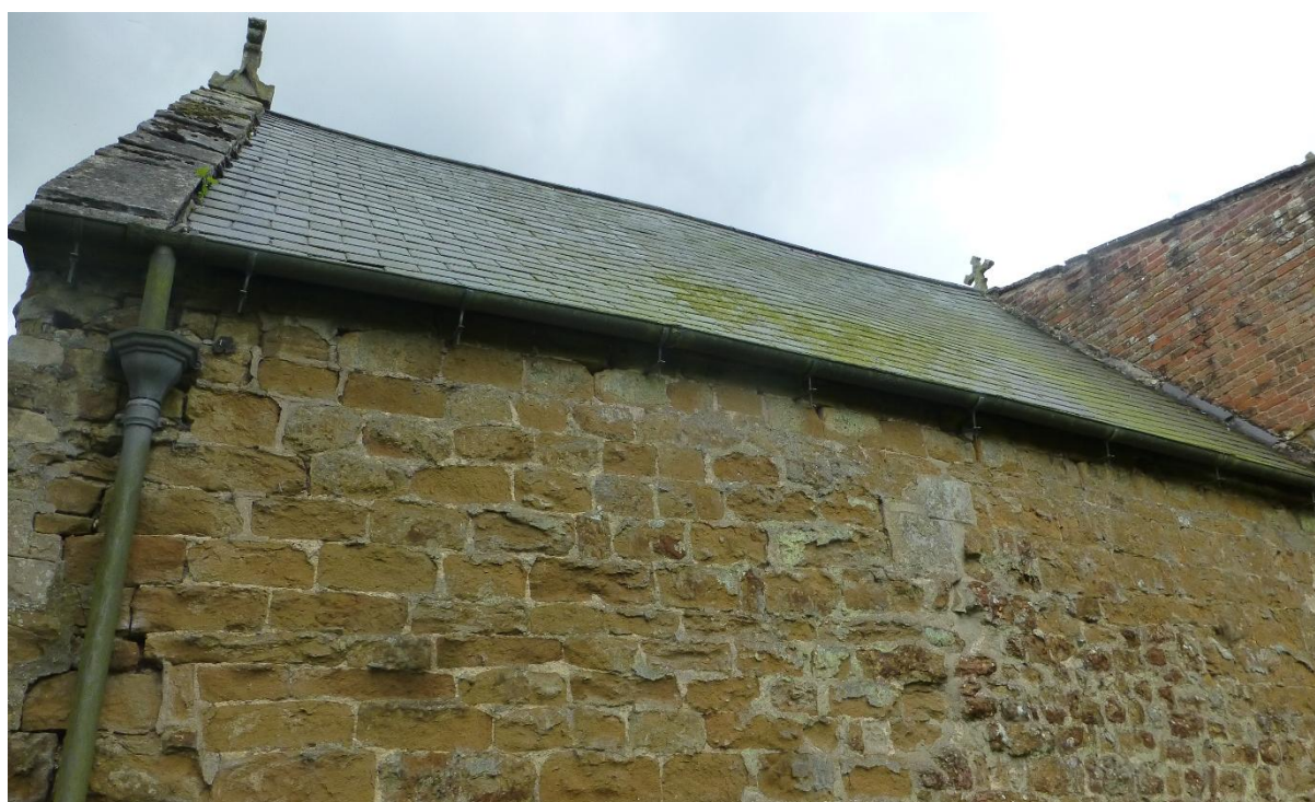
Photograph 10: North chancel wall with numerous gaps behind down pipe and below eaves
