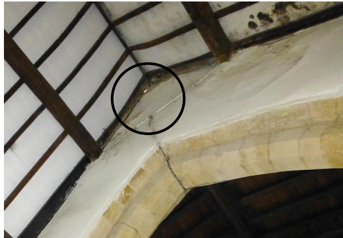
Photograph 7: Gap at apex of chancel roof and chancel arch
