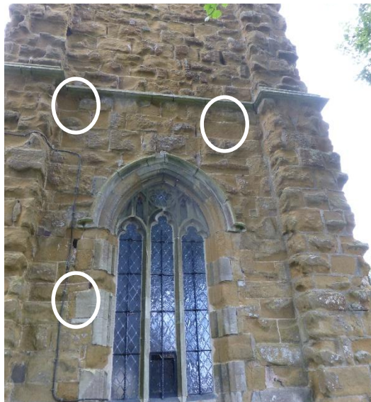
Photograph 11: West aspect of tower with gaps in stonework indicated
