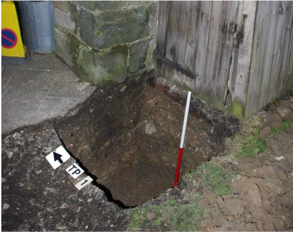
Figure 6 Fully excavated Test Pit 01 Tower foundations continue below base of test pit
