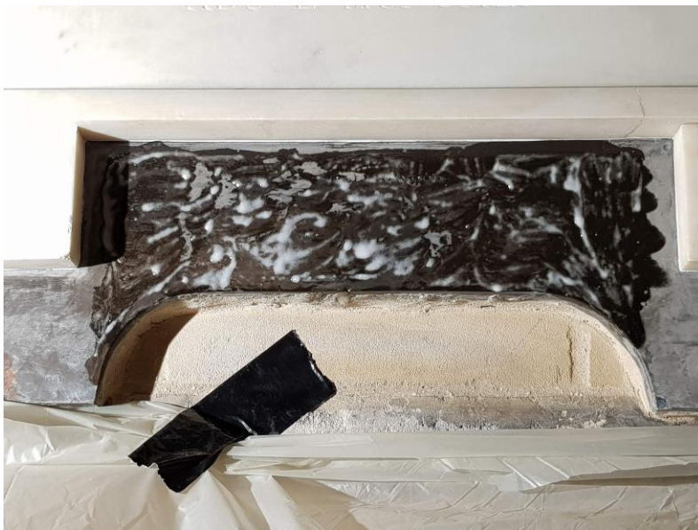
Figure 7: Image showing the poultice that was used on the black marble border.
