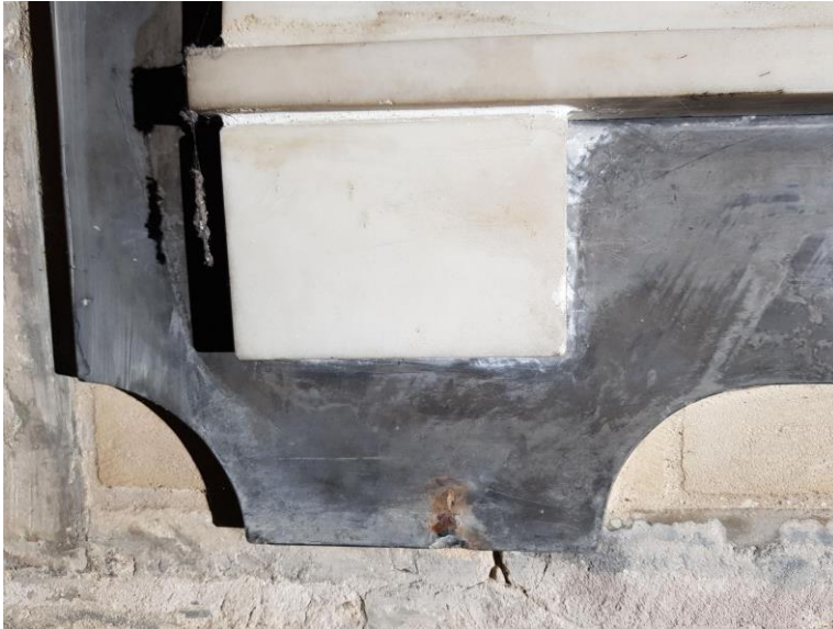
Figure 6: Rust stains on the monument to Georgiana Sibbeller Stevens.
