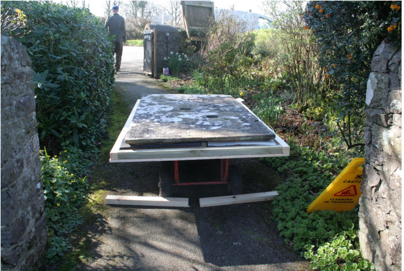
9 and 10. Removal of the slab – on the truck and below, the chest after removal of the slab, showing the prevalence of ivy
